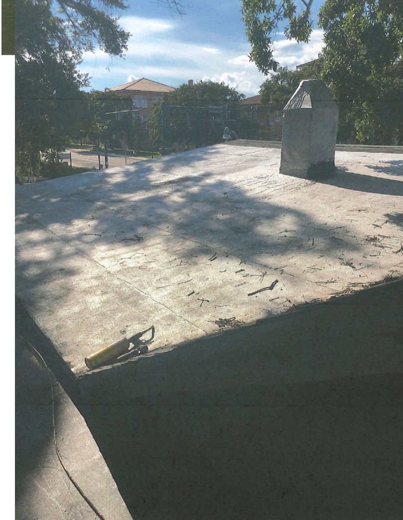
Pictures provided by the applicant showing the outside and inside damage caused by the roof leaks.
