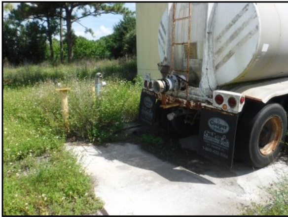
39 : Washwater transfer area to tanker trailer
