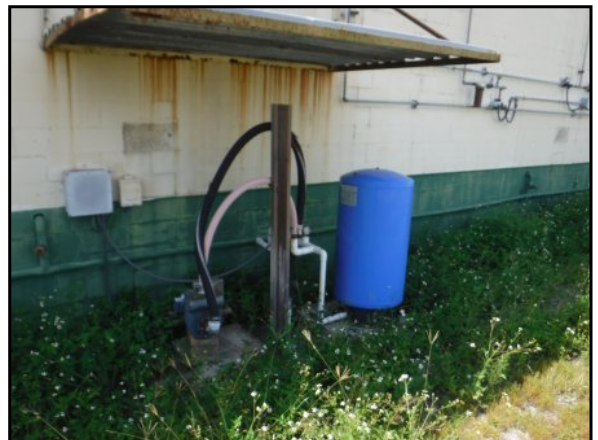
48 : Previous potable water well
