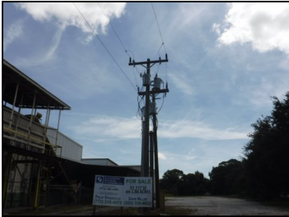
67 : Pole mounted transformers along southern adjoining street
