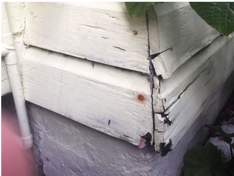
Existing —damaged siding. Pictures provided by the Applicant.
