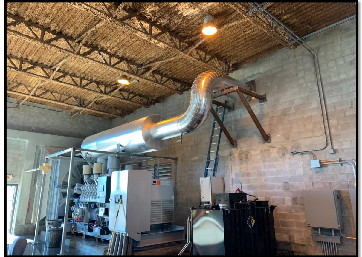
Completed and in-service MTU generator, day tank and exhaust piping. The generator and transfer switches are programmed to perform a test run for 4 hours every month.
