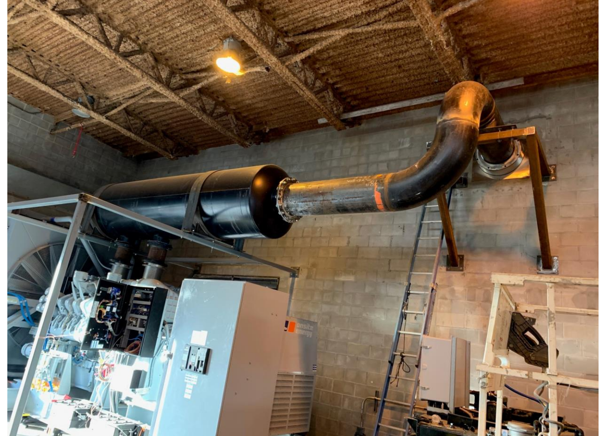
Exhaust piping being fitted and installed with outlet traveling through wall and up to atmosphere.
