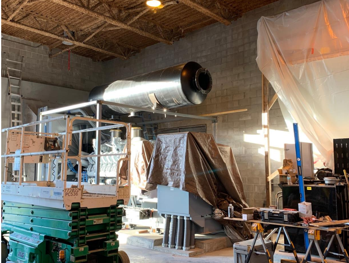
“Critical grade silencer” being installed onto generator exhaust manifold; final electric hookups between generator and transfer switches being completed.
