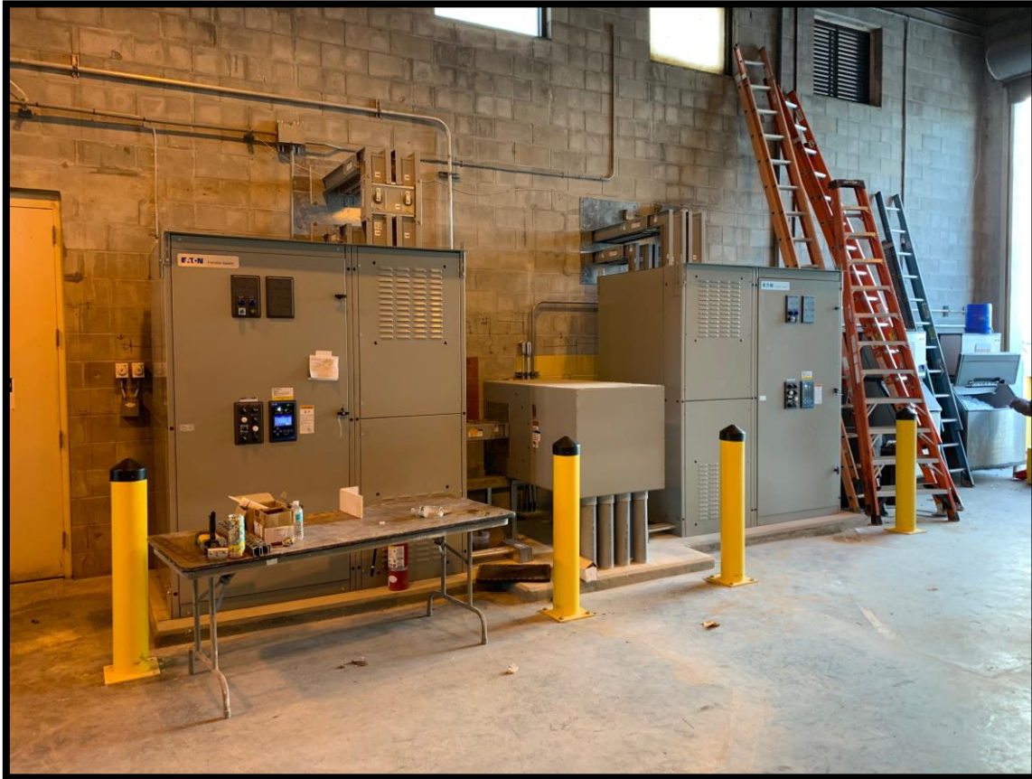
480 Volt Eaton Automatic Transfer Switches and new electrical busses installed and in service, protective bollards installed.
