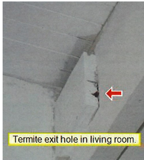
Interior damage pictures provided by the applicant
