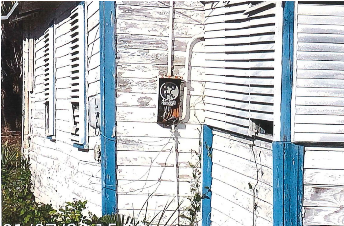
Exterior damage — pictures provided by the building inspector
