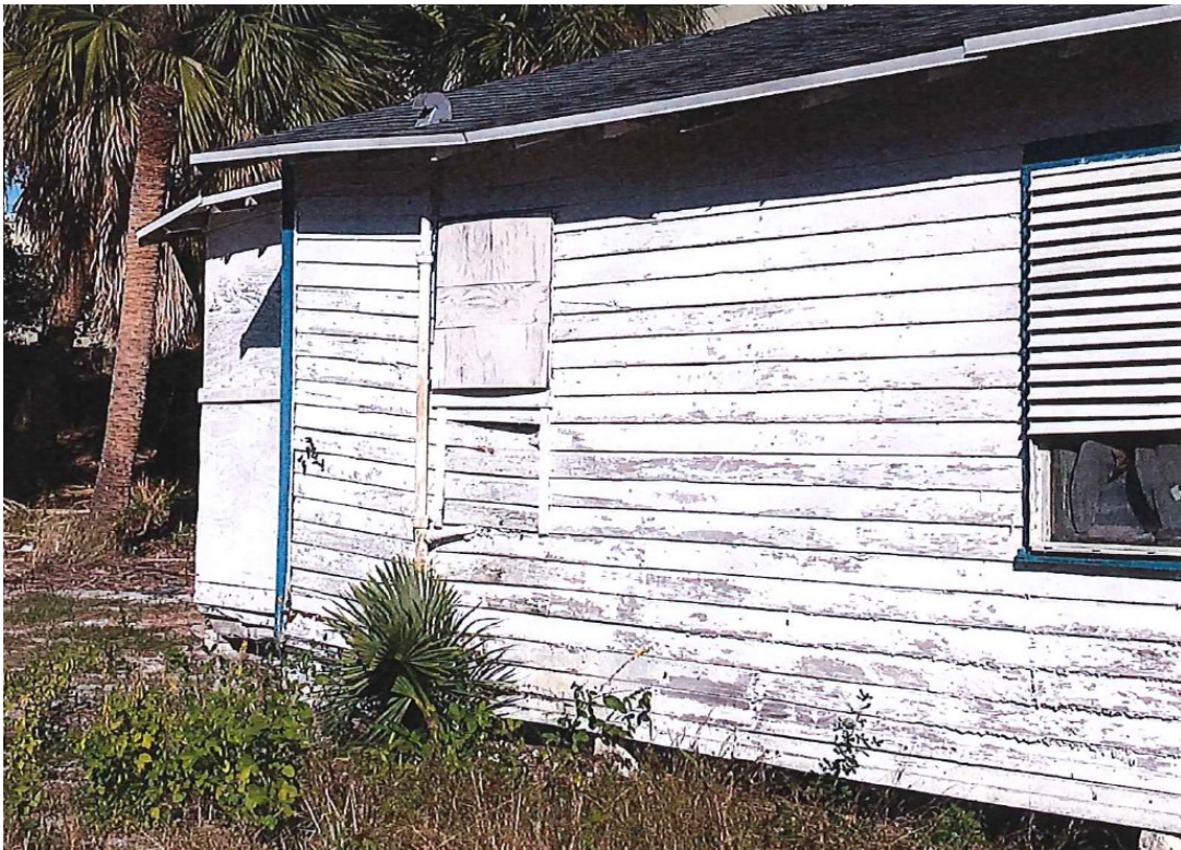
Exterior damage — pictures provided by the building inspector
