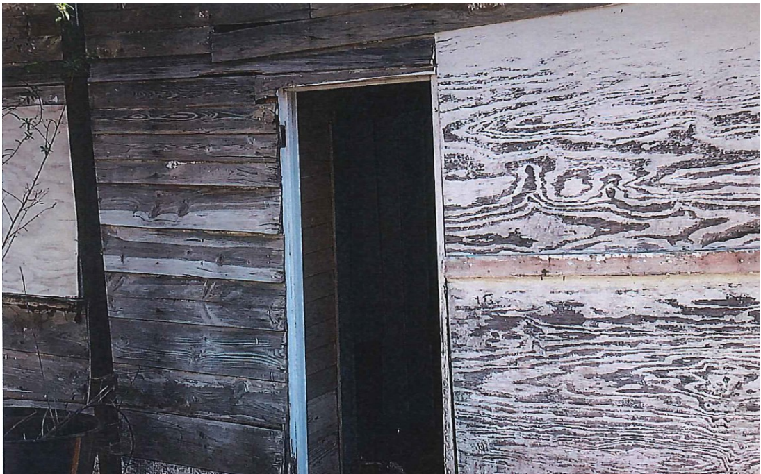
Exterior and interior damage — pictures provided by the building inspector
