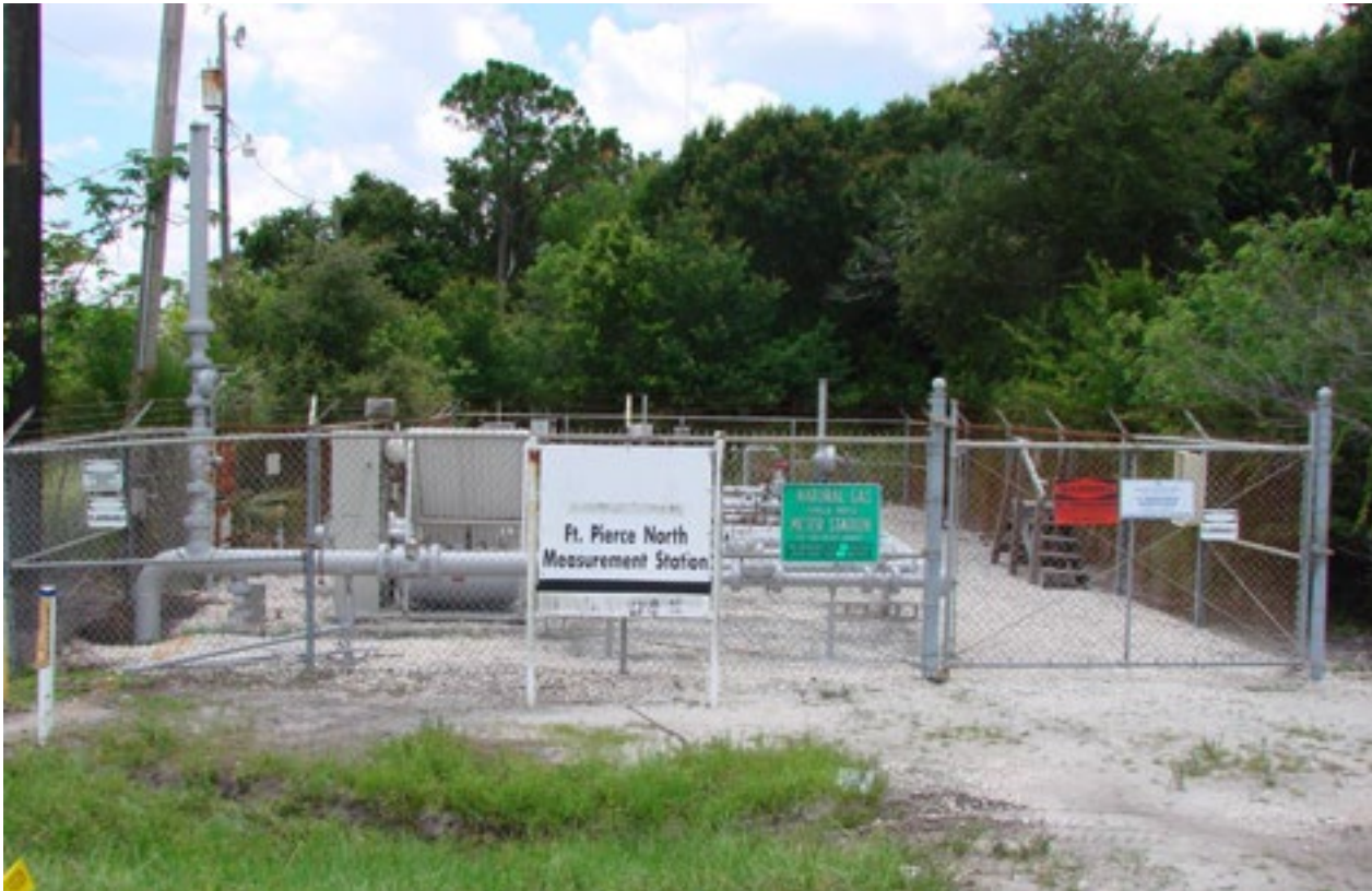
Fort Pierce Utilities Authority
