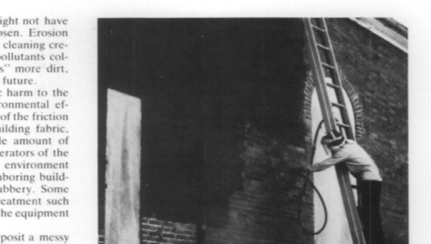
Abrading the Surface without Removing the Paint. Even though the entire outer surface layer of the brick has been sandblasted off, spots of paint still cling to the masonry. Sandblasting or other similarly abrasive methods are not always a successful means of removing paint.
