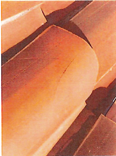
Cracked and shifted tiles noted throughout the field of the roof.
