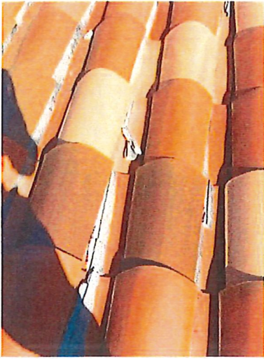
Tiles have shifted, mortar is no longer in place.
