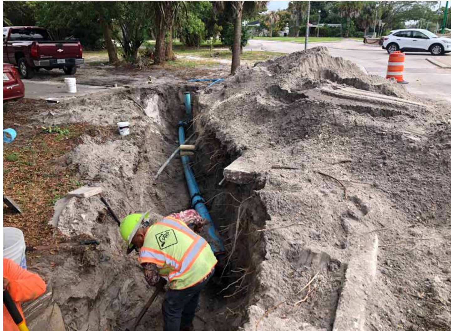
Potable Water Installation at Sunrise
