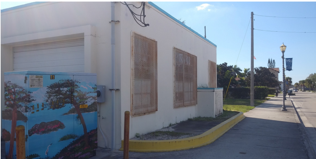
Exterior damage of the structure
