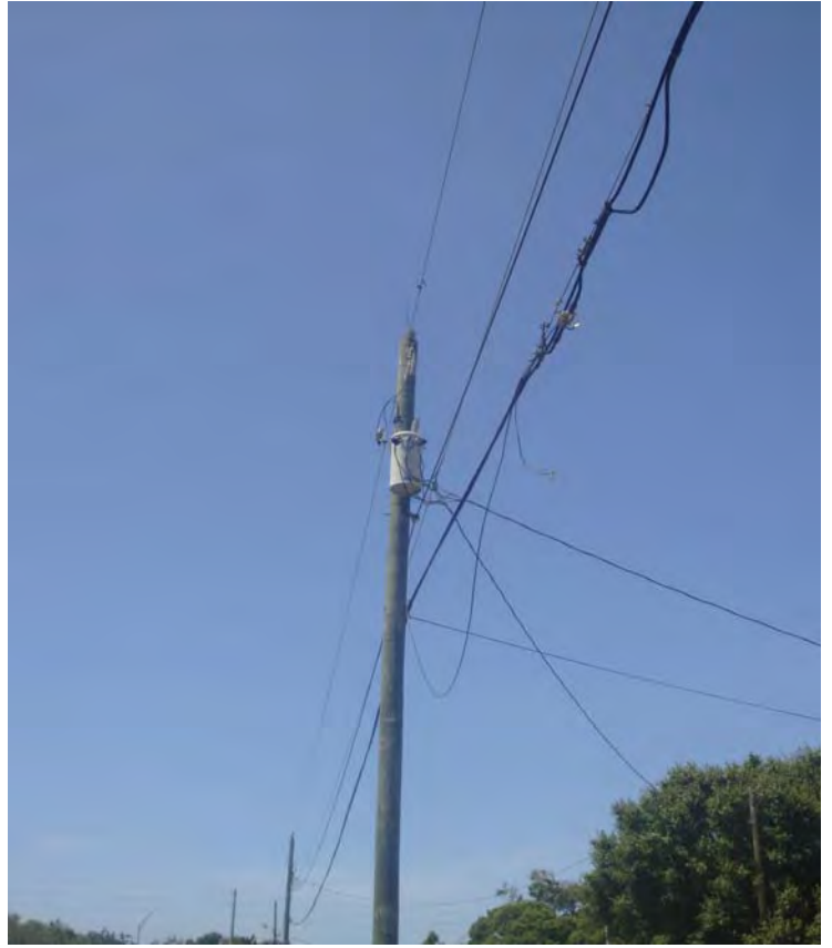
POLE MOUNTED TRANSFORMER
