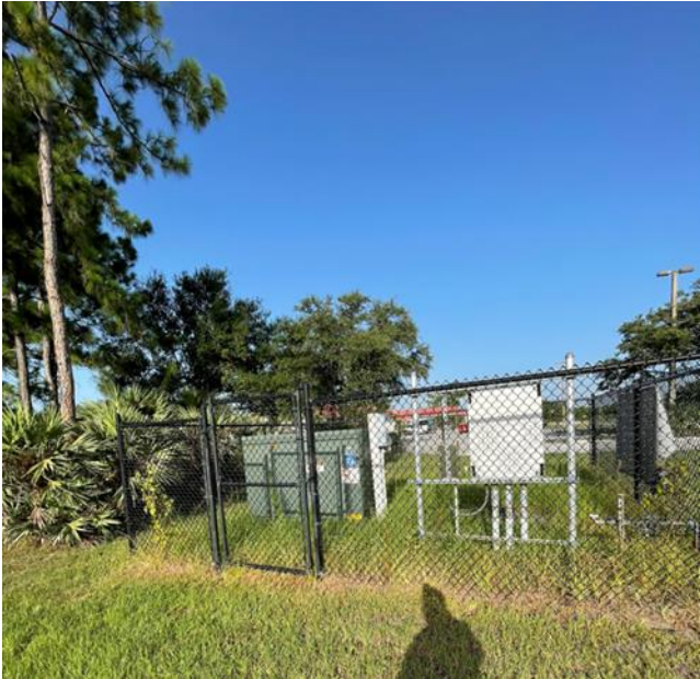
Figure 3 Fenced Electrical System on the southside of the property
