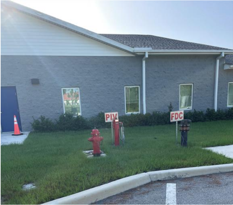
Figure 5 Fire Sprinkler System on south side of main building
