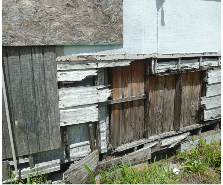
EXTERIOR DAMAGE OF THE STRUCTURE
