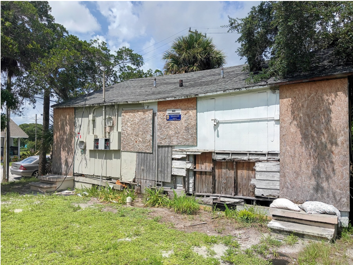
EXTERIOR DAMAGE OF THE STRUCTURE
