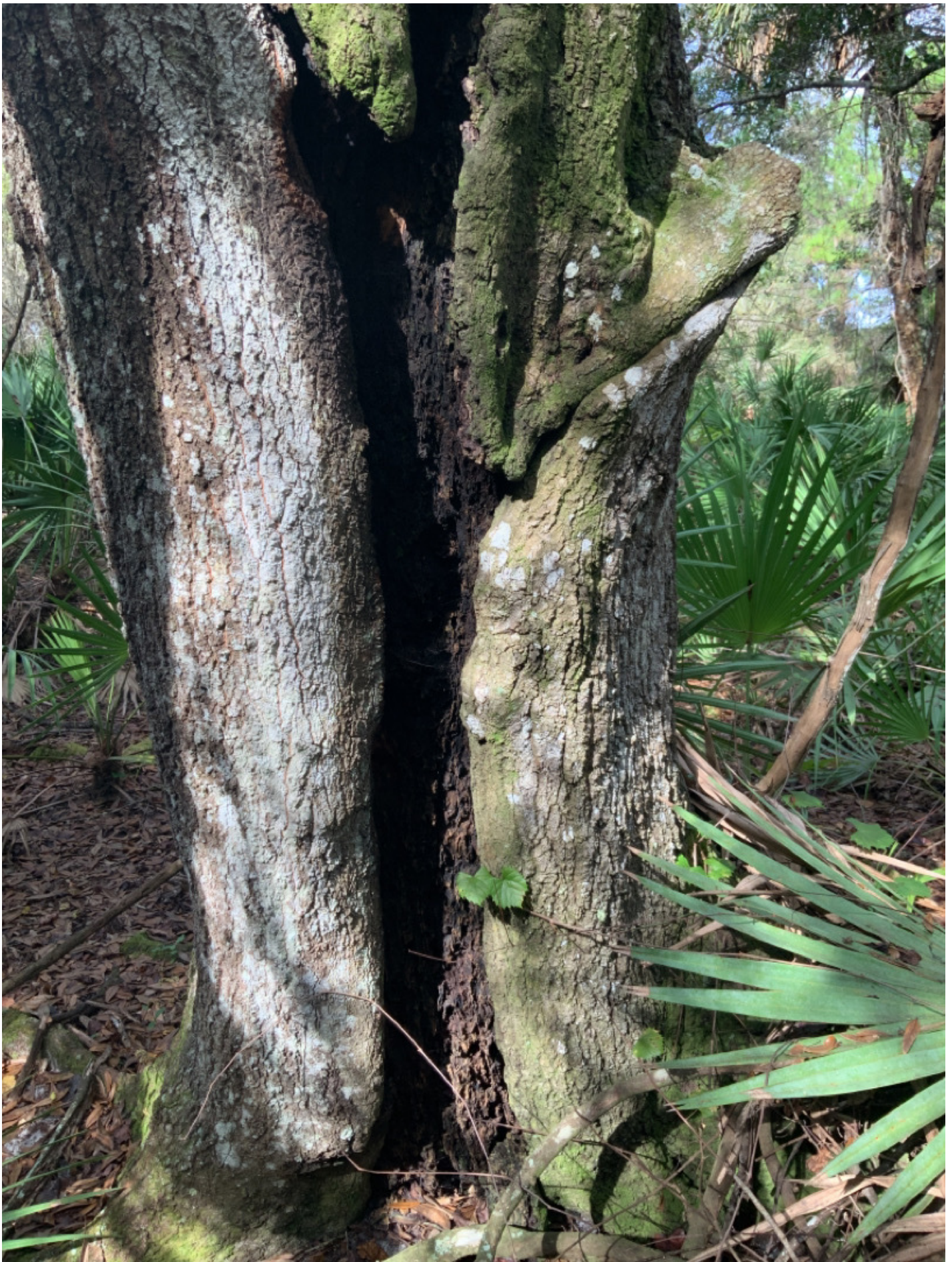
7. Tree 134 – hollowing and rot.
