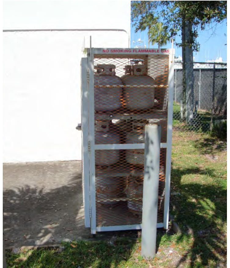
PROPANE TANKS AT SE CORNER OF COMMERCIAL BLDG.
