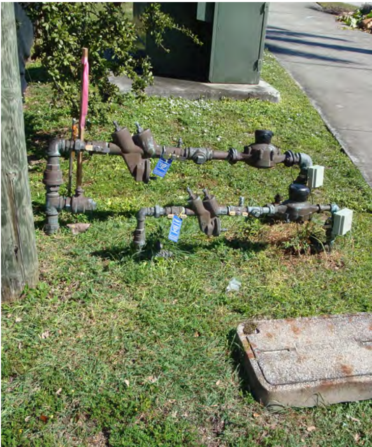
BACKFLOW PREVENTION AT SE CORNER OF SITE
