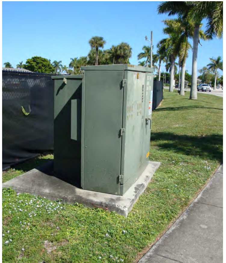
PAD TRANSFORMER AT SE CORNER OF SITE
