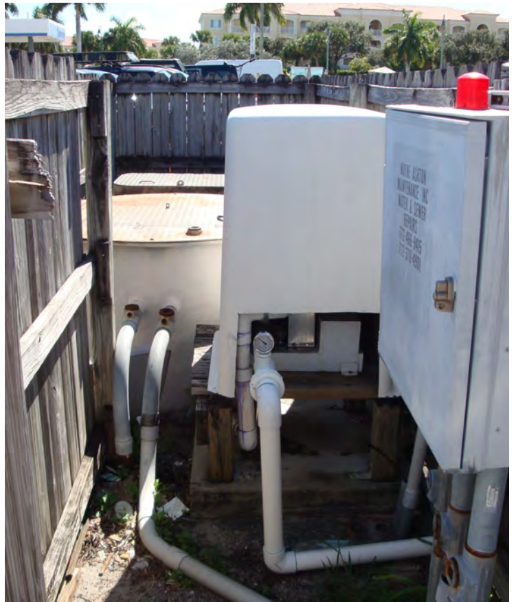
SEWER LIFT STATION
