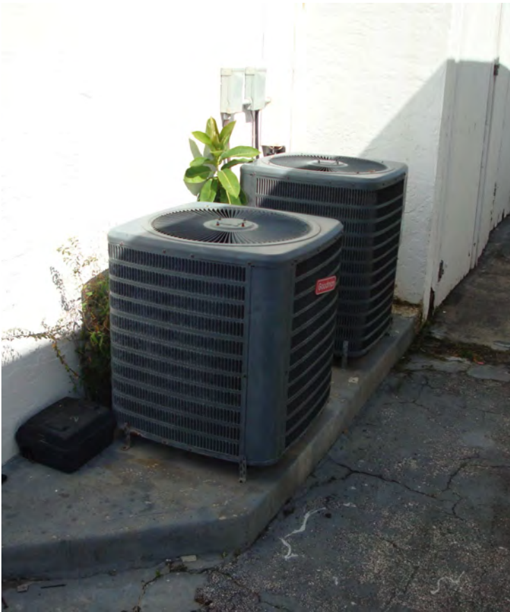
SPLIT SYSTEM HVAC UNITS
