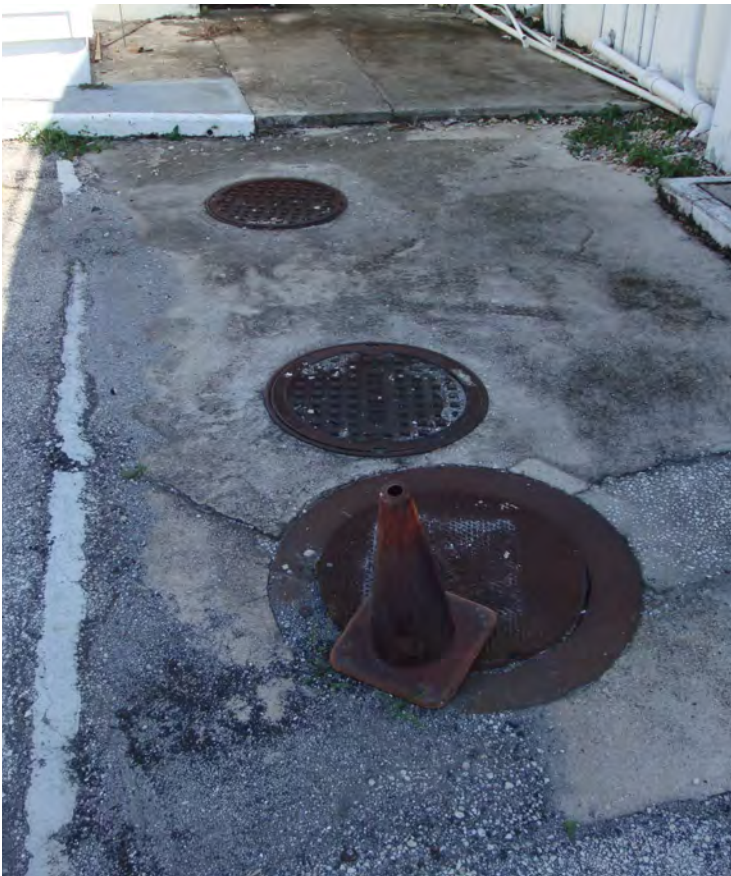
GREASE TRAP ON NORTH SIDE OF COMMERCIAL BLDG.
