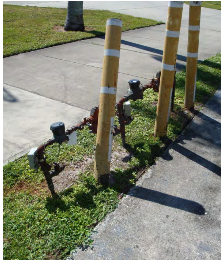
BACKFLOW PREVENTION ON SOUTH PROPERTY LINE
