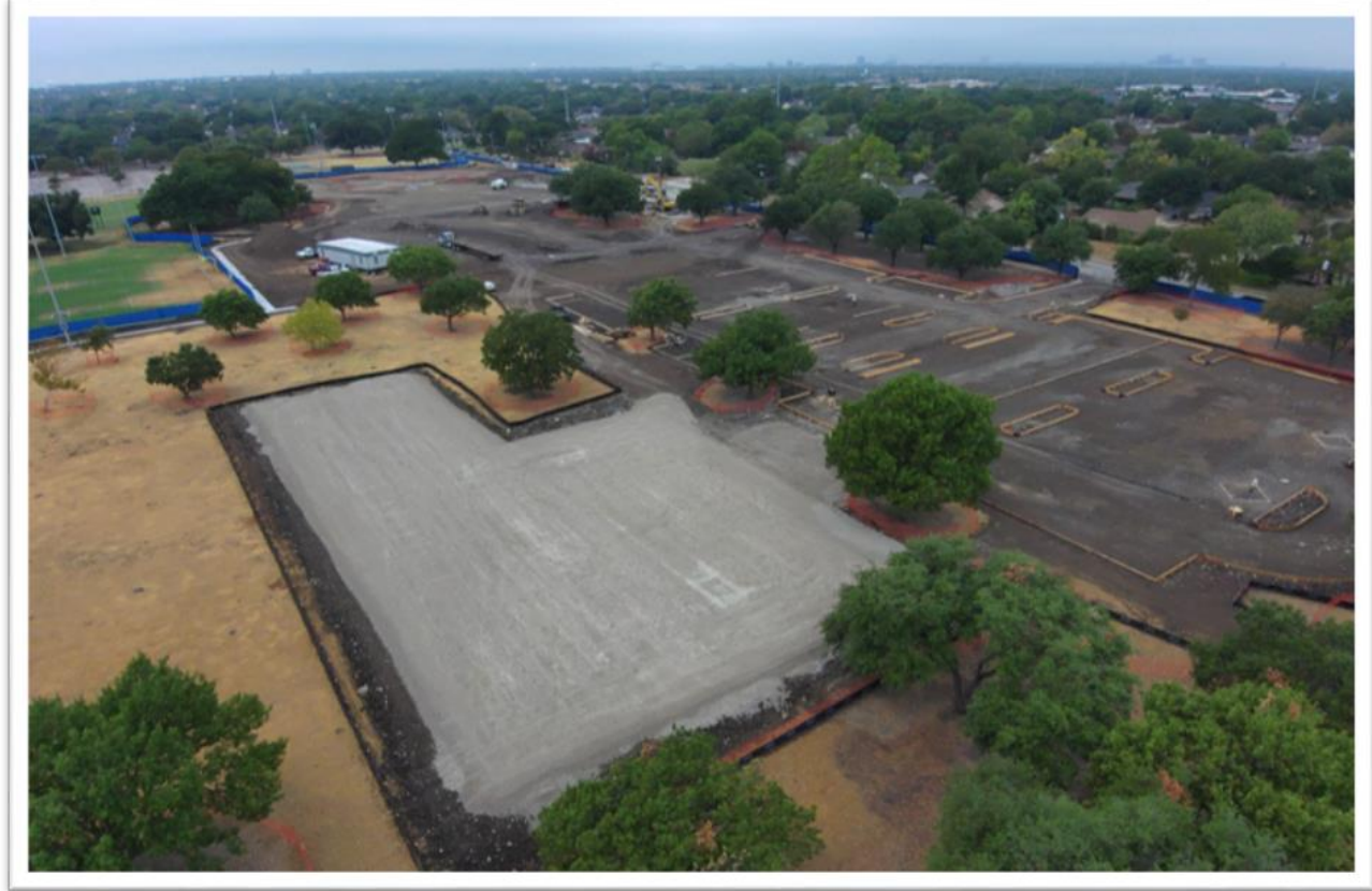
Construction progress photo – view looking to the northwest of future basketball and pickleball courts, parking lot
