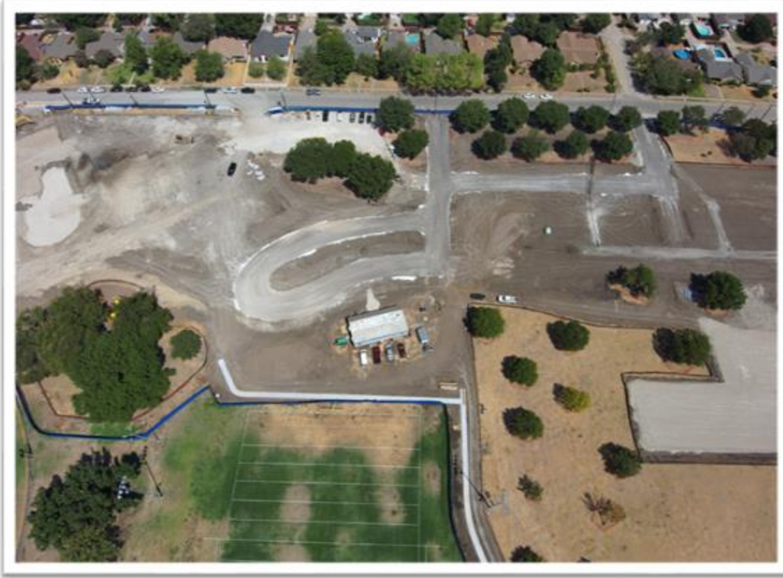
Construction progress photo – view of future recreation center, parking, and sports courts
