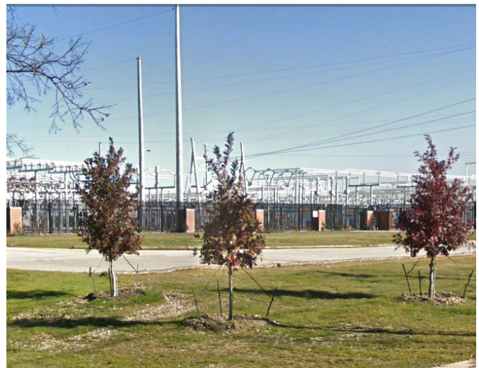
Substation (public/private utility) view at Telecom Parkway, north of Lookout Road
