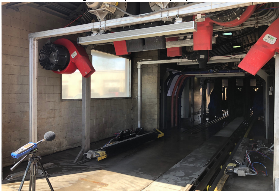
Figure 1: Sonny Blower-7 Dryer System
