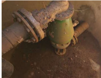
ARV Condition Photo 1
