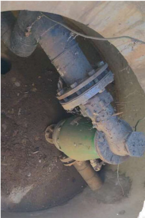
ARV Condition Photo 3
