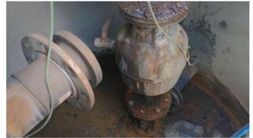
ARV Condition Photo 2
