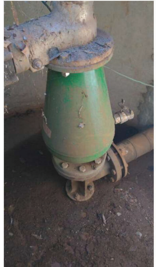
ARV Condition Photo 2
