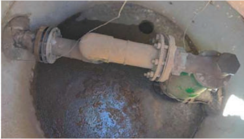
ARV Condition Photo 3
