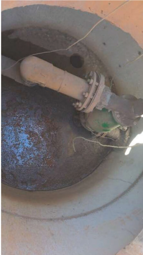
ARV Condition Photo 1
