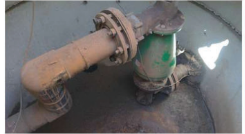
ARV Condition Photo 2
