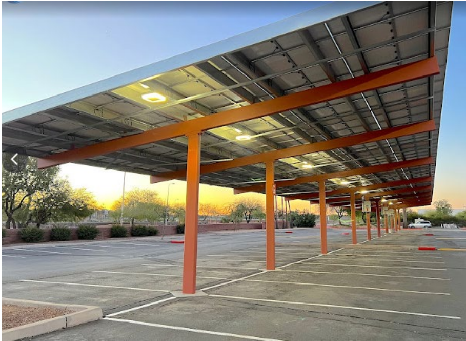
Solar Shade Structure with Cantilever Beam
