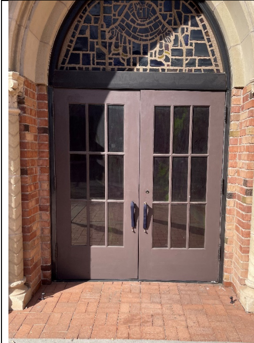
Main entry egress doors: Historic door pattern was uncovered, and hardware upgraded to current safety standards.
