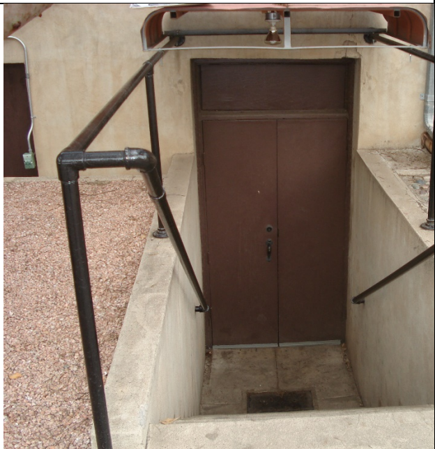
Basement railings and areaways: Conditions are hazardous and will be corrected in a compatible alteration of railings
