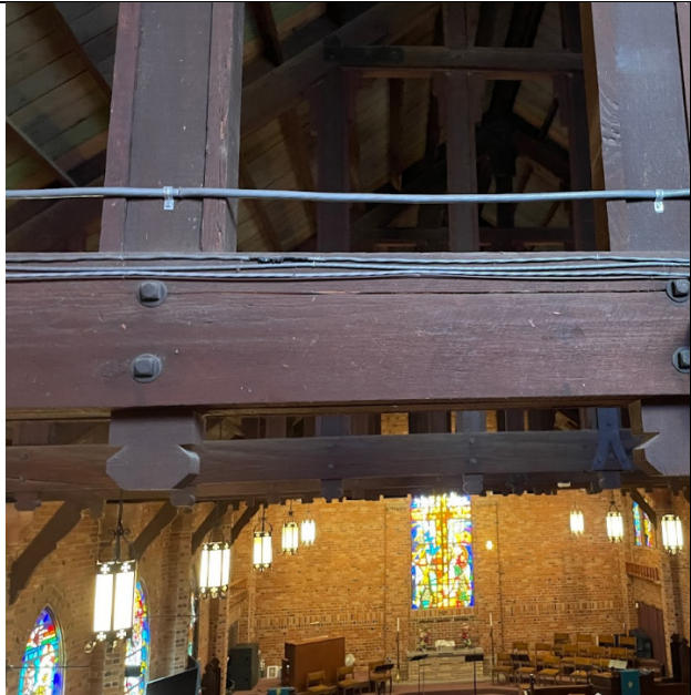
Wood roof trusses: Cracks in trusses reveal a failing condition requiring reinforcement
