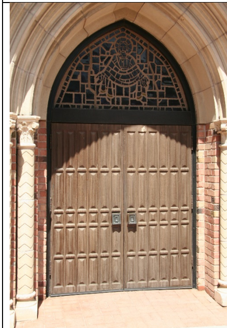
Main entry egress doors: Historic door pattern will be uncovered and hardware will be made safe
