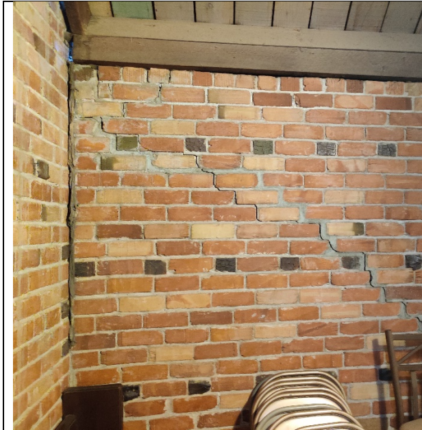
Structural brick repair and re-pointing: Brick walls have structural cracking in multiple locations
