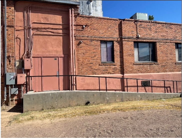
The handicap ramp in the back of the sanctuary was completely replaced to meet ADA requirements.
