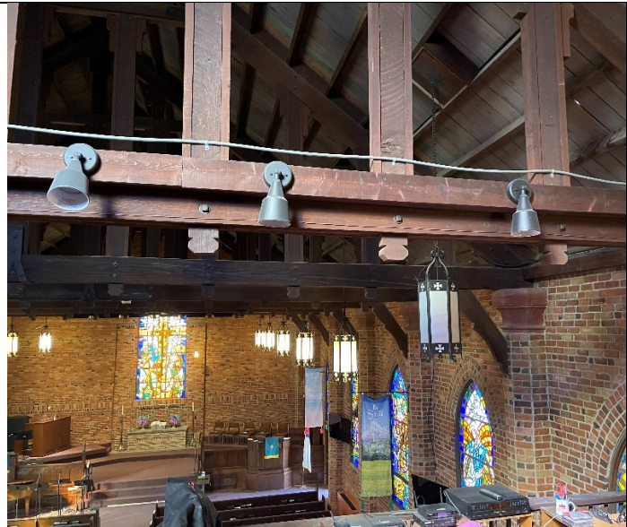
Wood roof trusses: Cracks in trusses revealed a failing condition requiring reinforcement. The wood roof truss pictured is reinforced and cracks in trusses have been restored.
