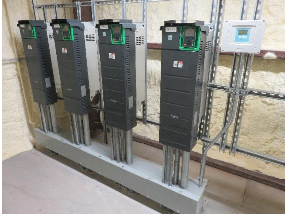
Links North Booster Station
