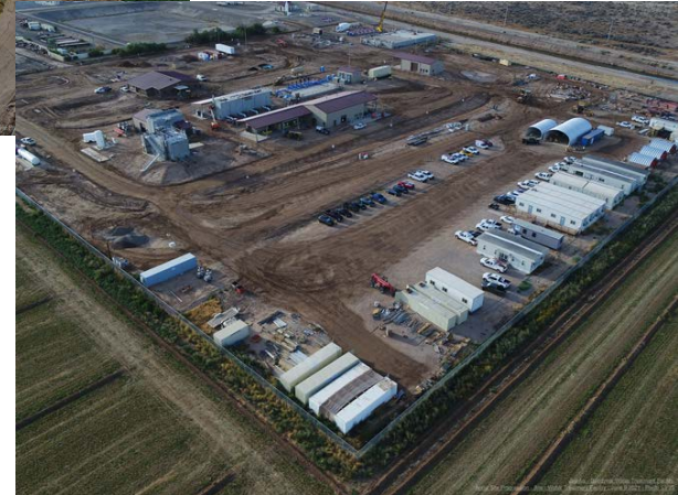
Surface Water Treatment Plant
