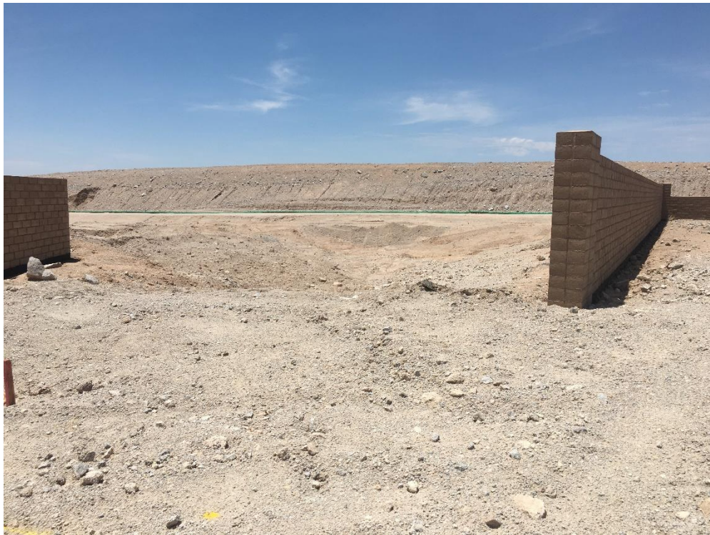
Looking west from near the west end of parcel 9.43, the large stack of dirt is off the property.
