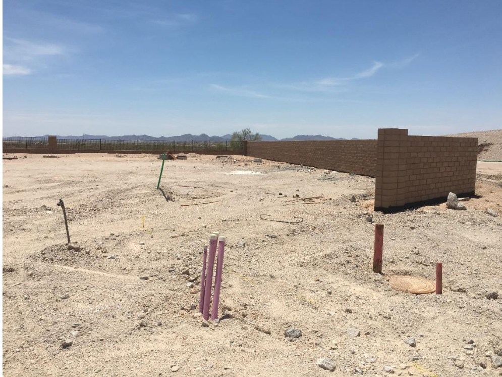
Another view of mostly finished perimeter slump block wall and wrought iron the fence.
