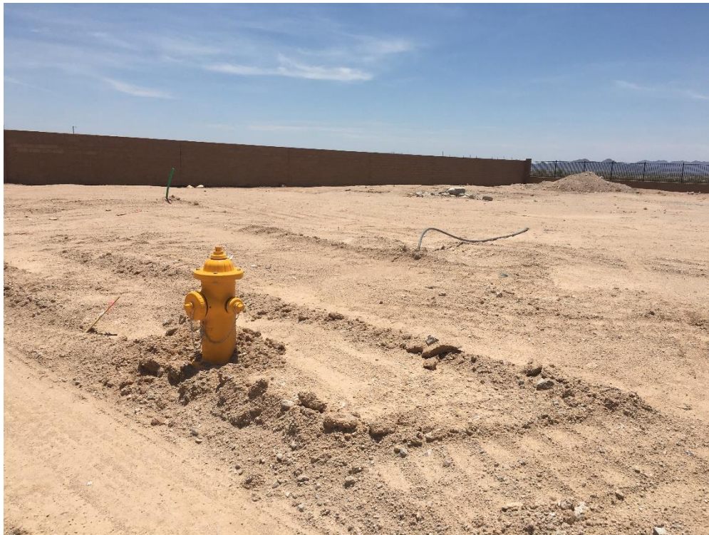
This fire hydrant reflects the finished condition of underground water and sewer lines.
