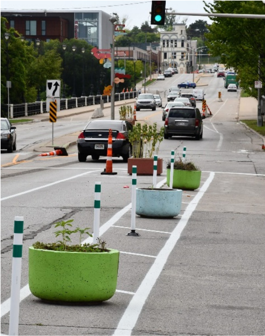
Exhibit 10. Quick-build pop-up Class IV bikeway created with planters, flexible posts, and striping (source: Urban Milwaukee)
