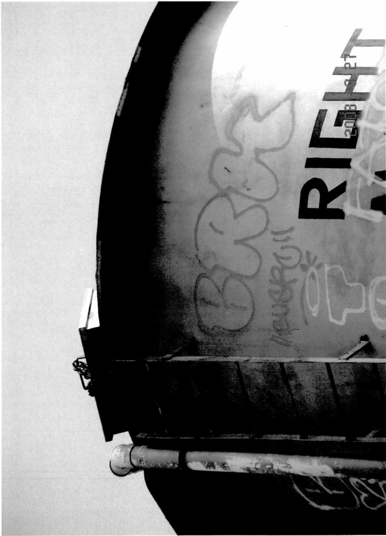
THIS PHOTO INDICATES INDIVIDUALS HAVE BEEN USING THE LADDER TO TAG ON THE WATER TOWER.
