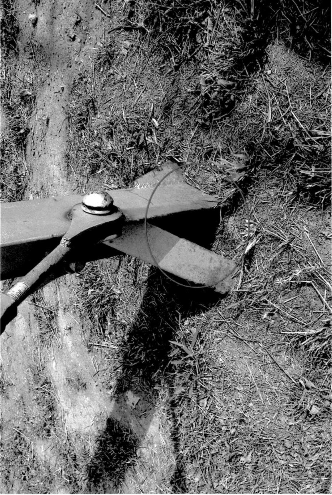
THIS PHOTO SHOWS THE ANCHOR BOLT IS MISSING A NUT.
