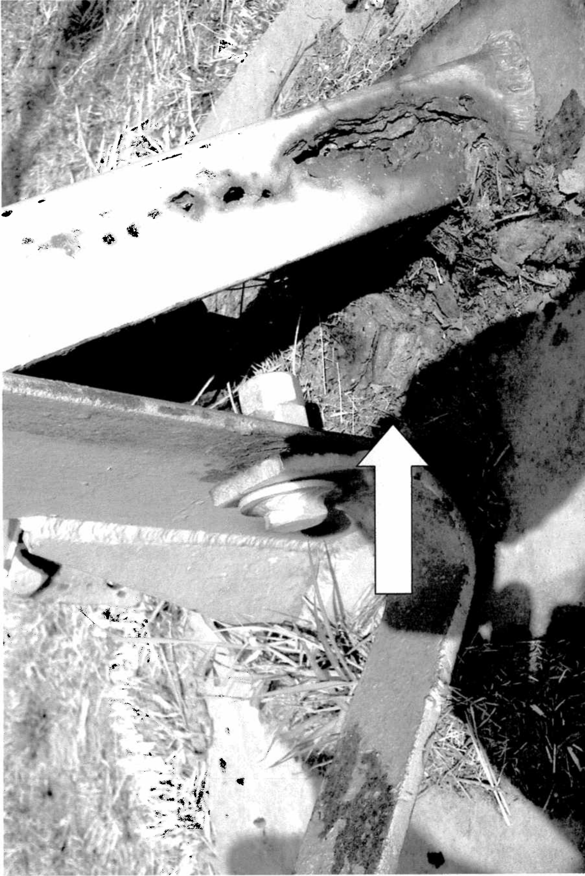
THIS PHOTO SHOWS THE CONDITION OF AN ANCHOR BOLT THAT HAS BEEN SEVERLY AFFECTED BY CORROSION.
