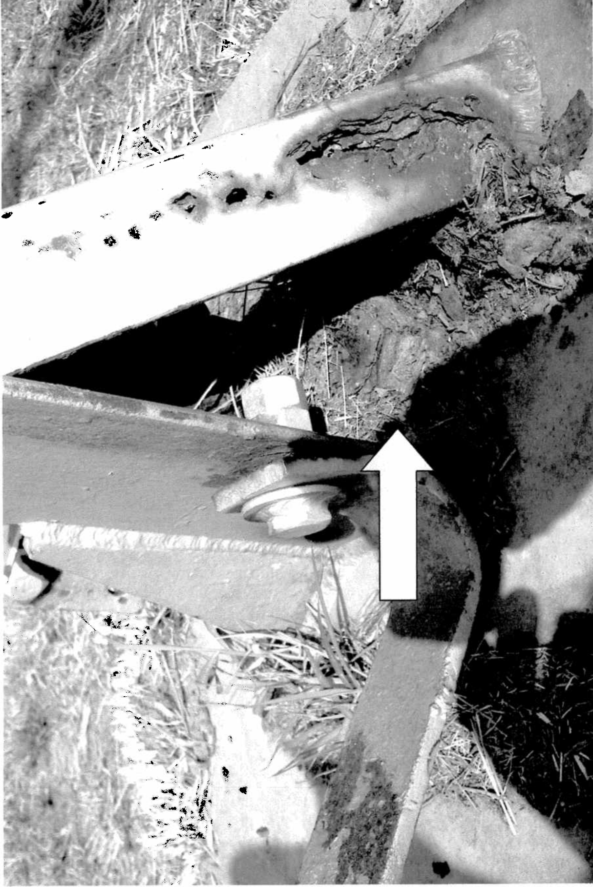
THIS PHOTO SHOWS THE CONDITION OF AN ANCHOR BOLT THAT HAS BEEN SEVERLY AFFECTED BY CORROSION.
