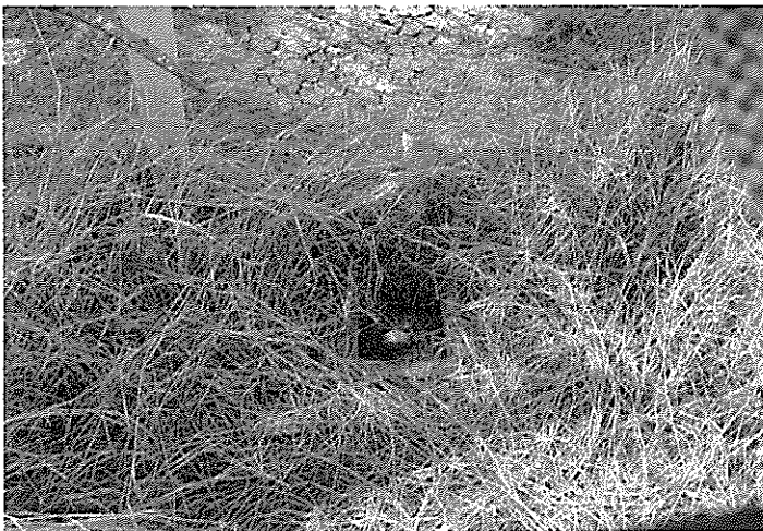
Photo 7 Western view of water meter located along the part to be acquired.
