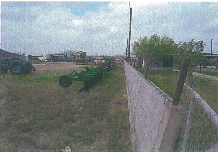
Photo 7 Western view of block fence located within the part to be acquired. It appears the wall is leaning at a 80 degree angle and is supported by the chain link fencing.
