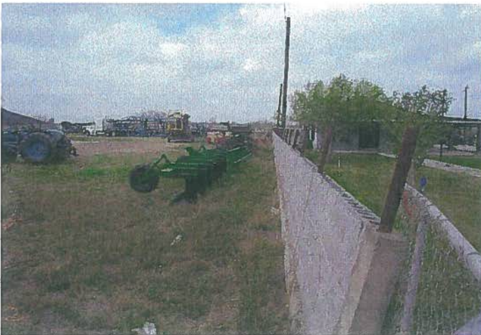
Photo 7 Western view of block fence located within the part to be acquired. It appears the wall is leaning at a 80 degree angle and is supported by the chain link fencing.
