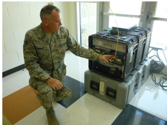
Texas State Guard demonstrates the wireless internet router and the land line telephone for the satellite communications system
