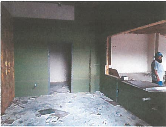
Moisture resistant dry-wall at kitchen.
