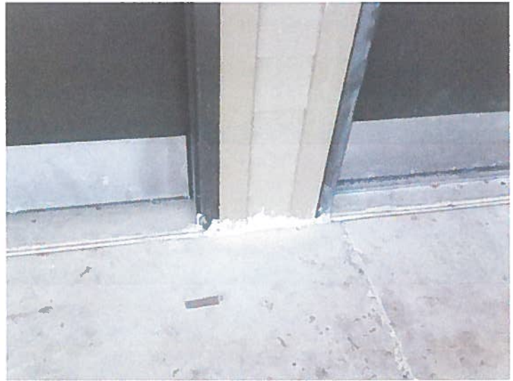
spatter on exterior walls
