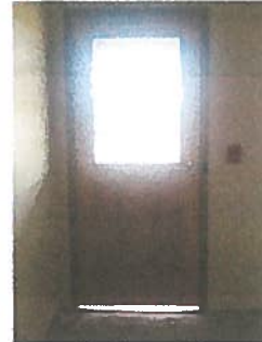
Gap at bottom of door.
