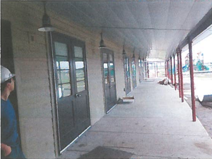
Lights along corridor
