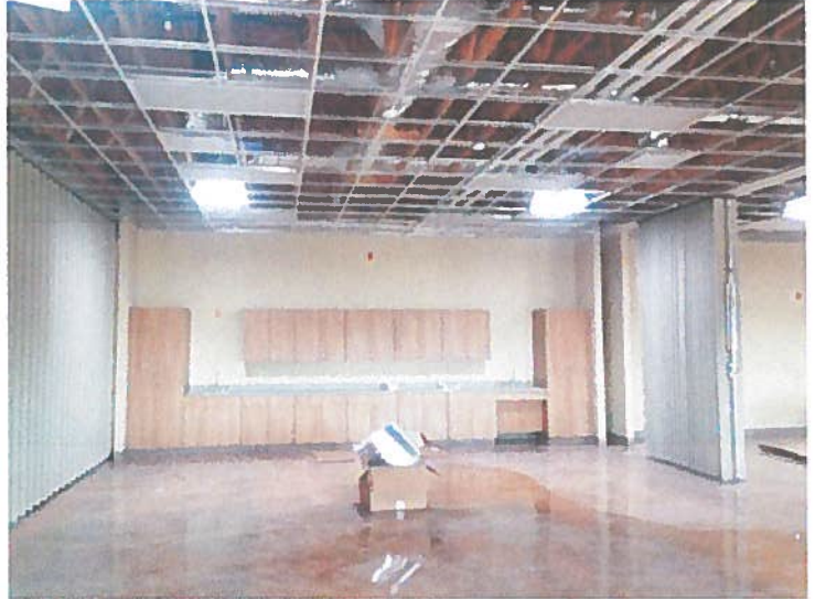
solatubes at Multipurpose
