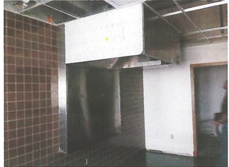
kitchen vent hood at kitchen
