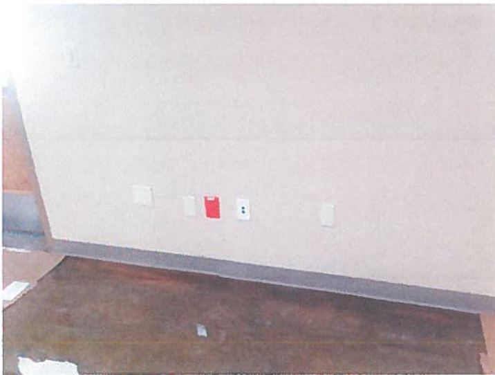
Outlets not in-line
