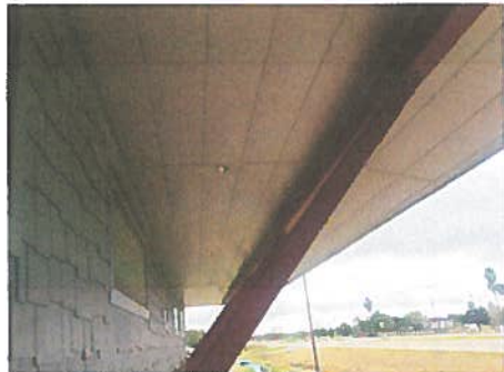
Oil-canning at soffit needs corrective work.
