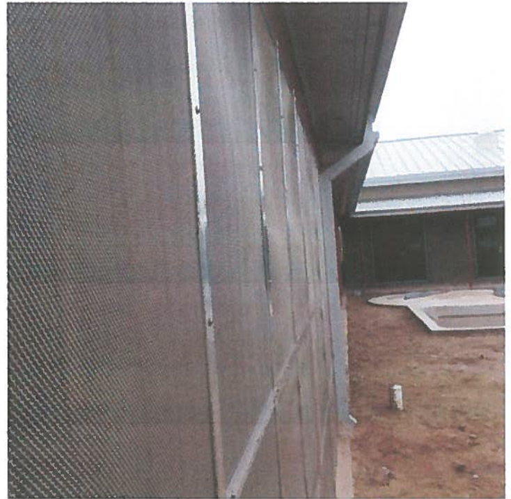
Mesh screen, screws not in line
