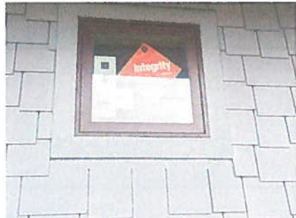
Siding piece needed below windows.
