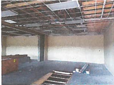
Multi-purpose Room, no electrical power.
