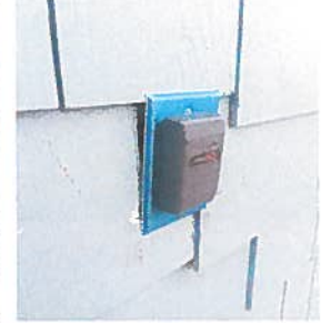
Installation not acceptable.
