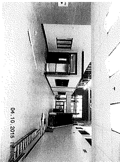
Atrium: Walls painted 95%, doors & windows installed, floor tile installed. General clean out in-progress.
