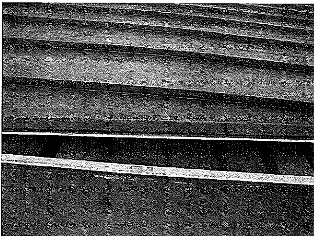
Snap lock panel is easily removed. No underlayment present. Metal panels are installed directly to the metal deck.
