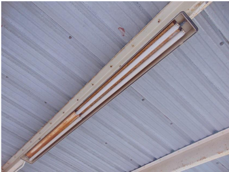
Some fixtures need replacing
