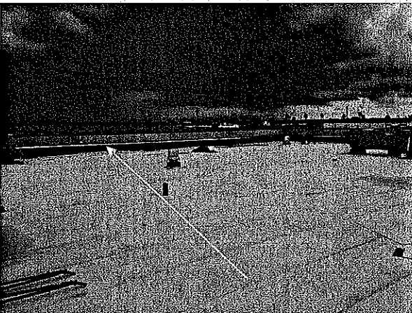
Tinsmiths continued installing the sheet metal reglet onto the walls of Kitchen Maintenance.
