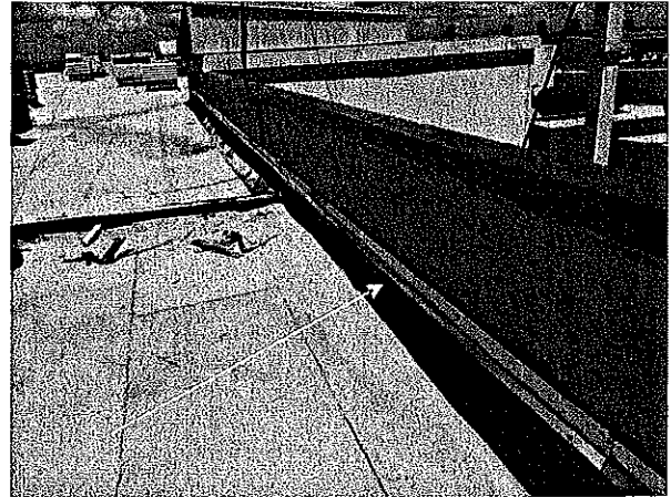
Tinsmiths began installing the sheet metal reglet onto the parapet walls of Fox roof.
