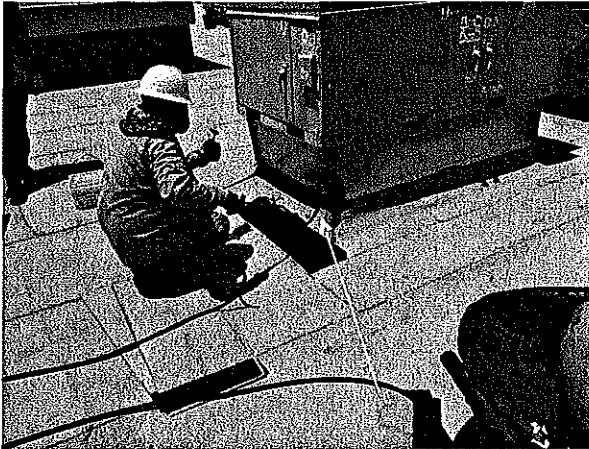
Roofers began installing the modified base flashing to the mechanical curbs on Fox roof.
