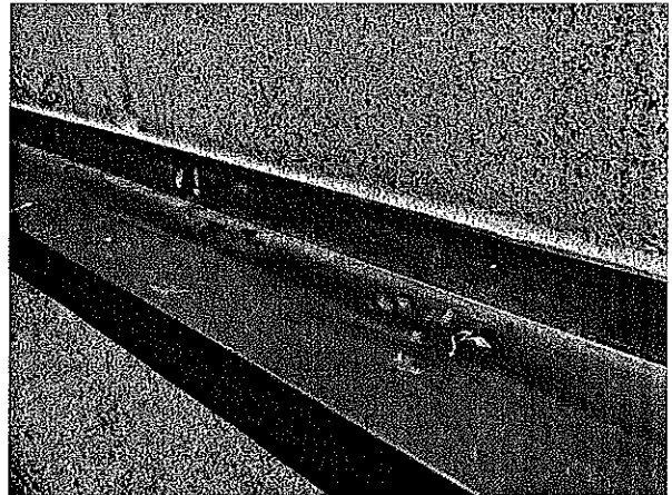
The top half the cap was fitted over the bottom half and anchored to the intersecting wall.
