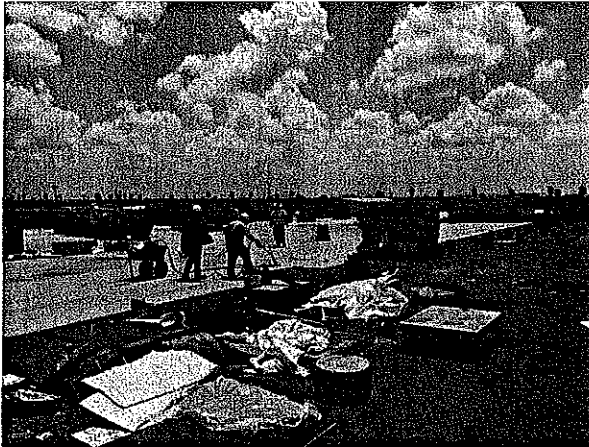
Roofers continued installing the cap ply across the field of roofs Gulf & Kitchen Maintenance.
