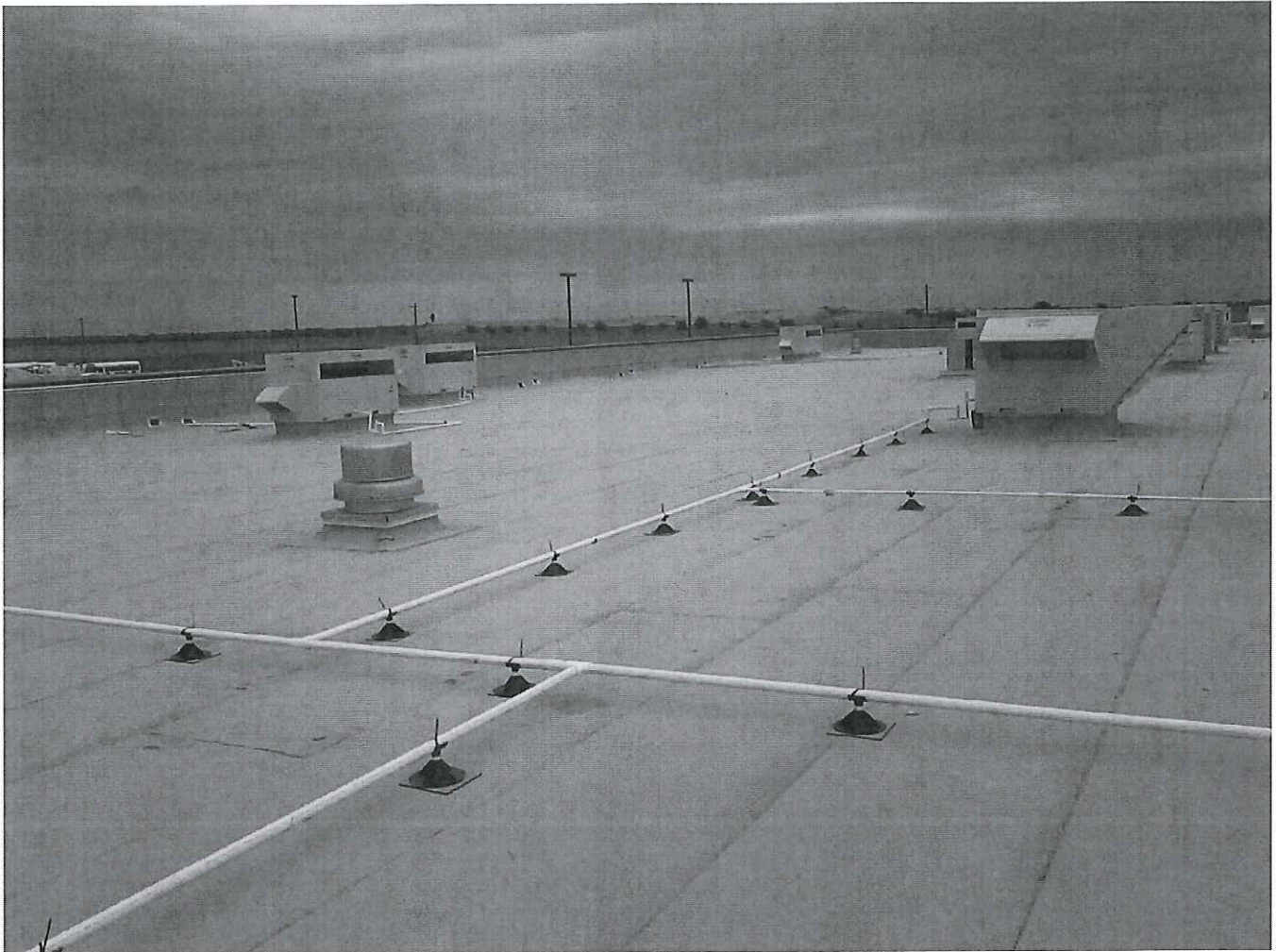
Condensate lines throughout the roof
