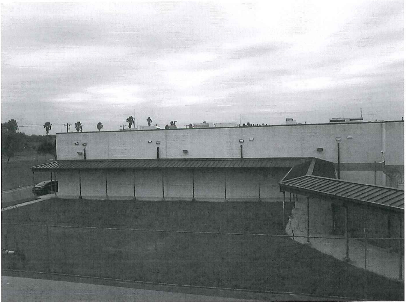
Unfinished head scuppers at the ADC
