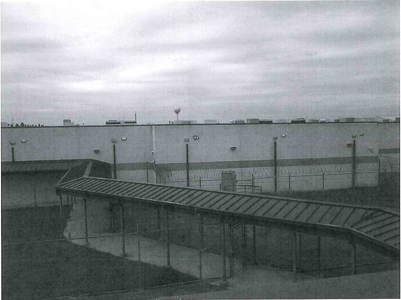
Unfinished head scuppers at the ADC
