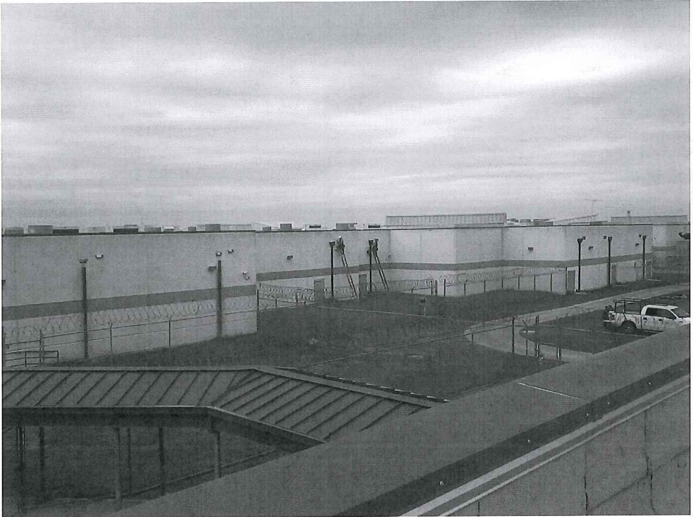
Contractor working on the head scuppers at the drains at the ADC
