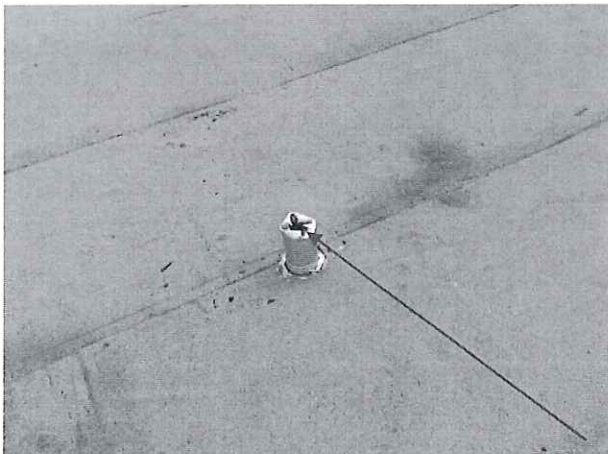
Properly fold the top of lead jack into the pipe on the Kitchen Maintenance roof.
