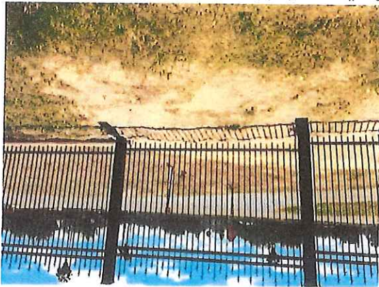
Grading near the intersection of Hwy 107 and Sunflower Road had been modified by county crews during the installation of the perimeter fencing, creating an area of water retention.
