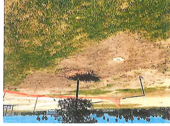
Grass removed | scraped-off during the excavation of the plumbing lines by county crews. Landscaper will not need to replace the grass.
