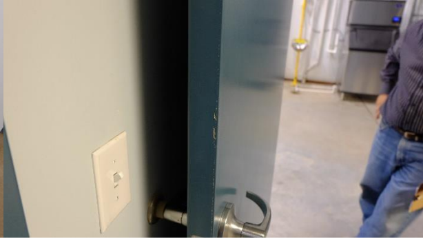
4.16 Patch cracks in door. Re-finish as needed.
