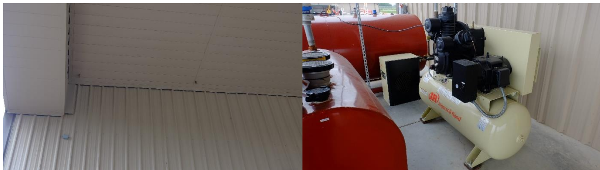
4.1 Pre-engineer metal brackets missing.
