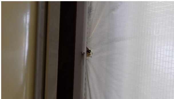
4.31 Patch all damaged insulation liner.
