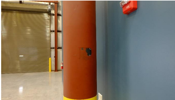
4.17 Paint damaged crane system columns.
