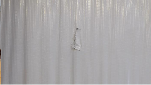
4.34 Patch all damaged insulation liner.
