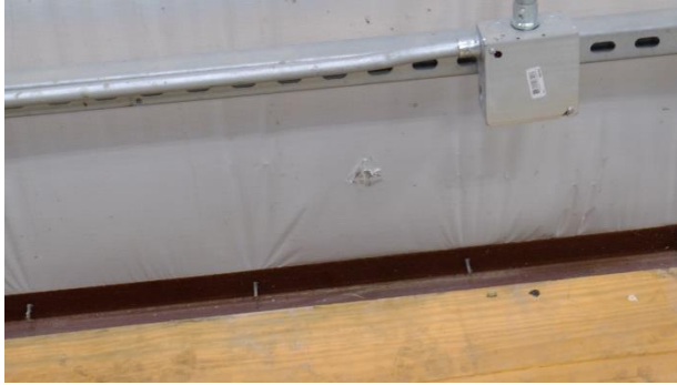
4.33 Patch all damaged insulation liner.
