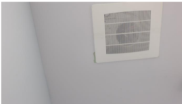
4.37 Paint scuff marks by exhaust fan on shower room.
