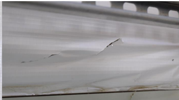
4.32 Patch all damaged insulation liner.
