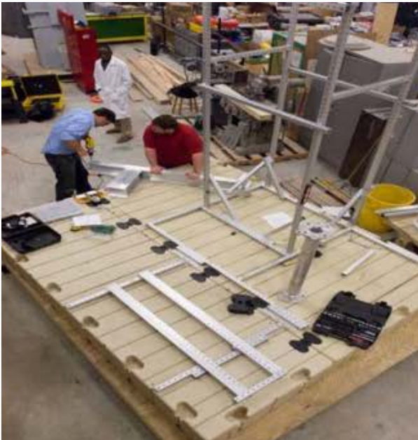
Figure A5 Construction of moored robotic platform in "Old Main" high bay
