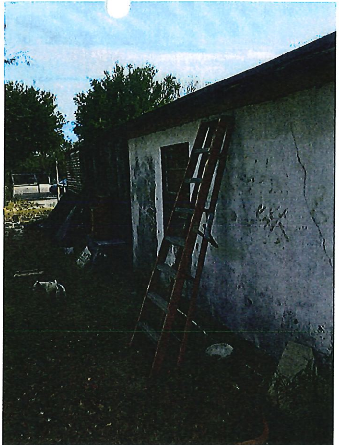
North Side of Home. Trim And Soffit Damage
