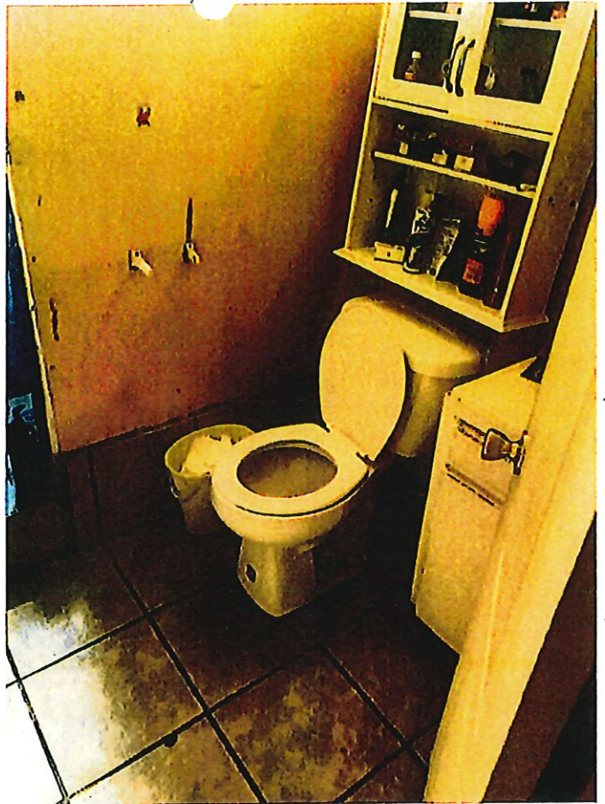
Toilet in Bathroom Not functioning properly. Low water pressure
