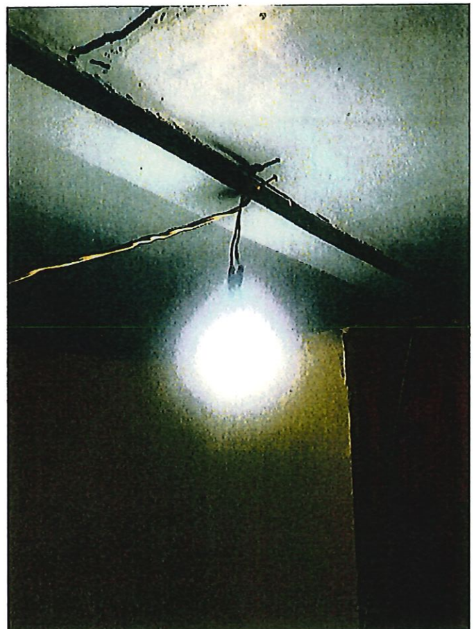
Hanging light with extension cord.
