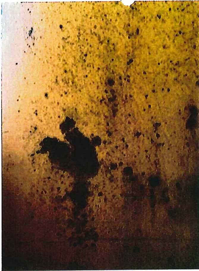
Looks like mold located in Bathroom.
