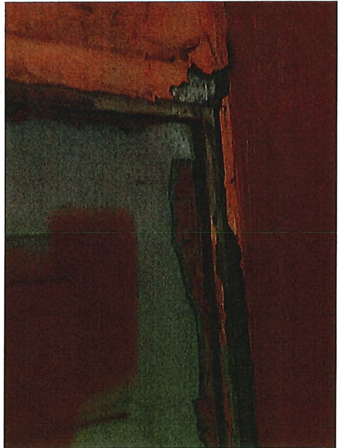
Damage to Bathroom Door
