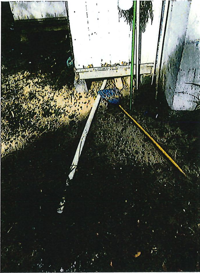
Exposed plumbing draining to the yard.
