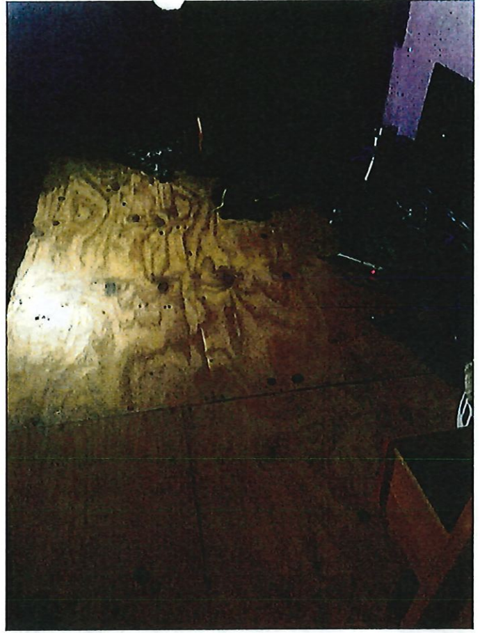
No flooring in bedroom #2. Exposed plywood decking.
