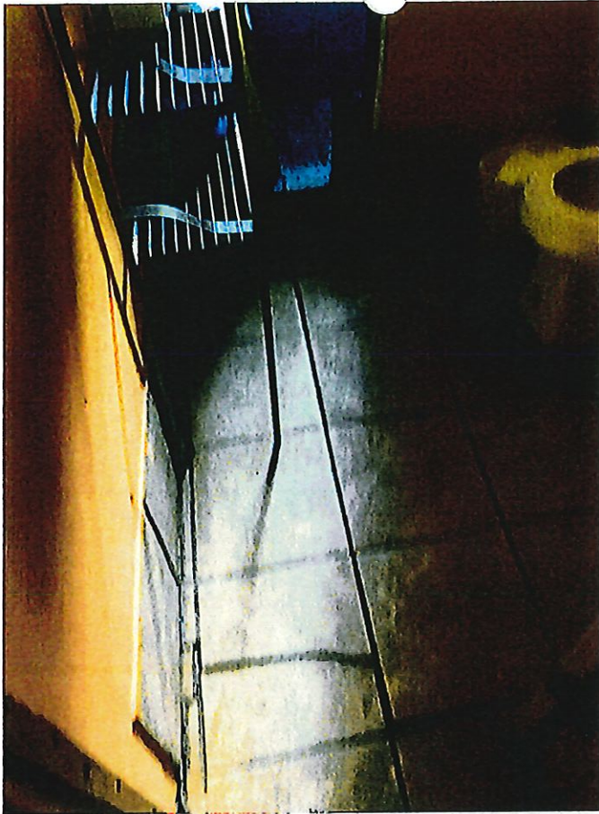
Ceramic tile in Bathroom Cracked due to Subfloor Movement
