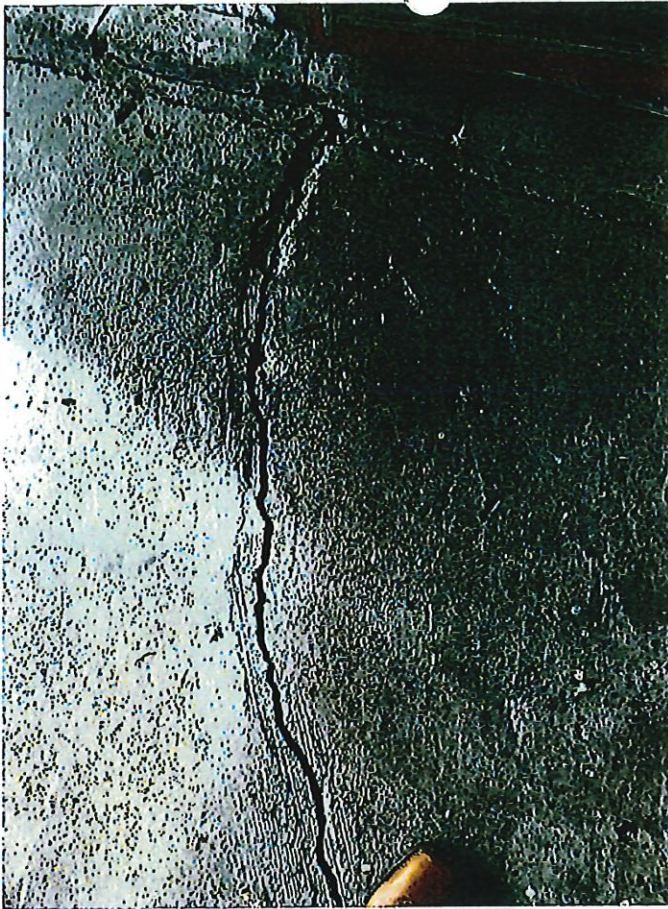
Crack located on front porch
