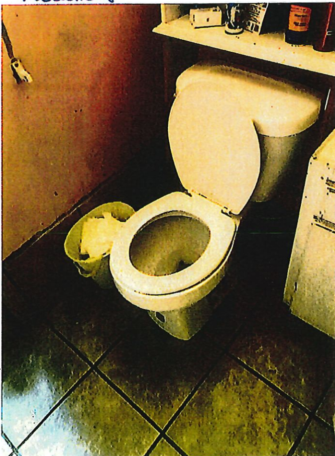
Cracked ceramic tile beneath the Toilet.
