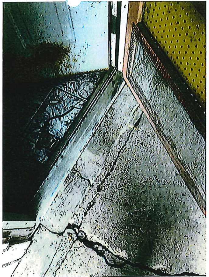
Large crack in front porch By front door HAZZARD.
