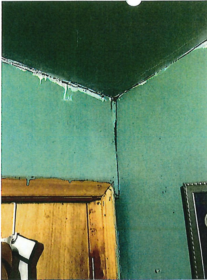
Large crack in wall by master Bedroom door.
