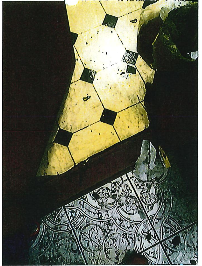
Entry to master bedroom. Tripping hazard.
