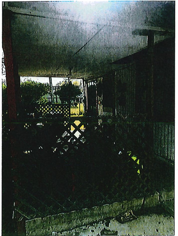
front porch, concrete floor is cracked.
