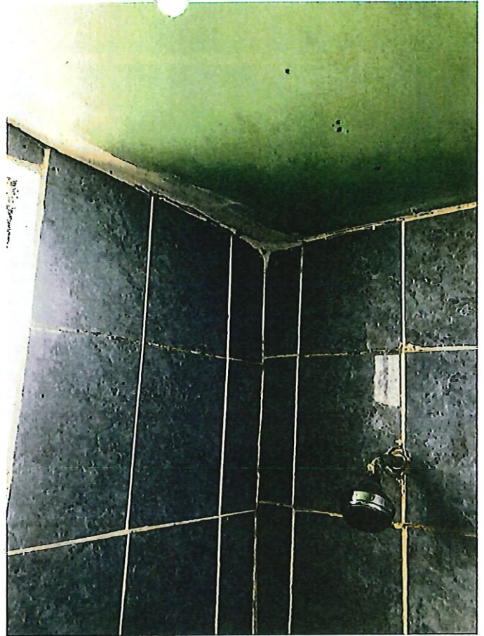
Shower head broken
