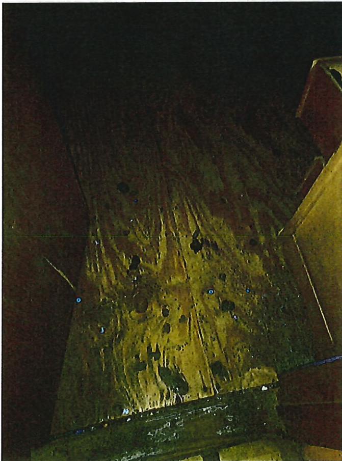
Entry to bedroom #2. Exposed Plywood decking.
