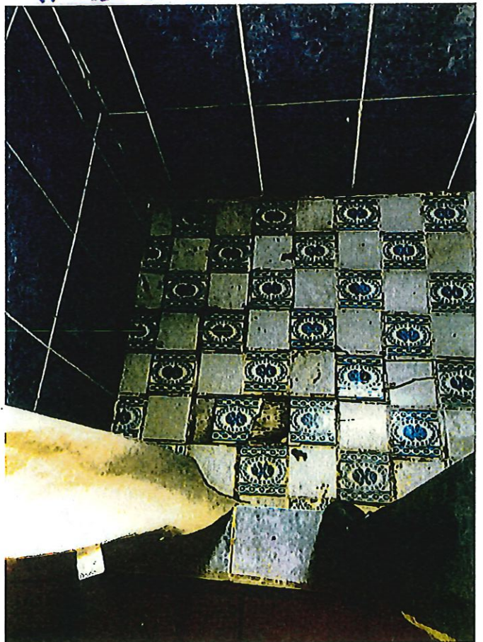
Broken tile in shower.
