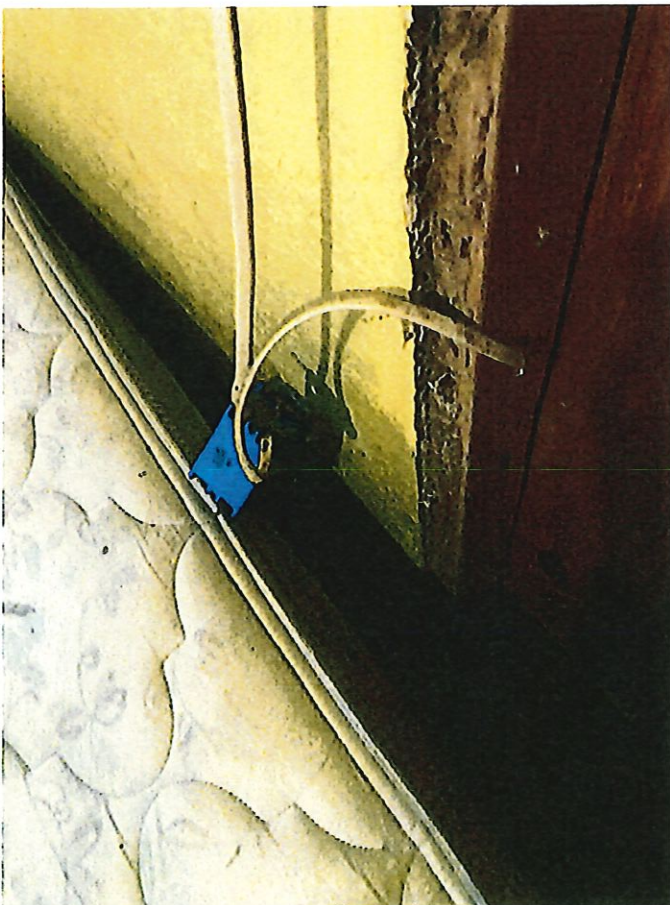
Exposed Electrical wiring and wall over next to bed.
