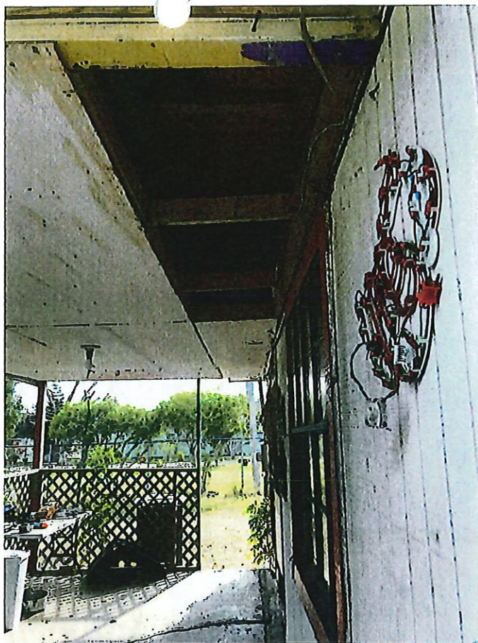
Plywood Soffit in porch area missing.
