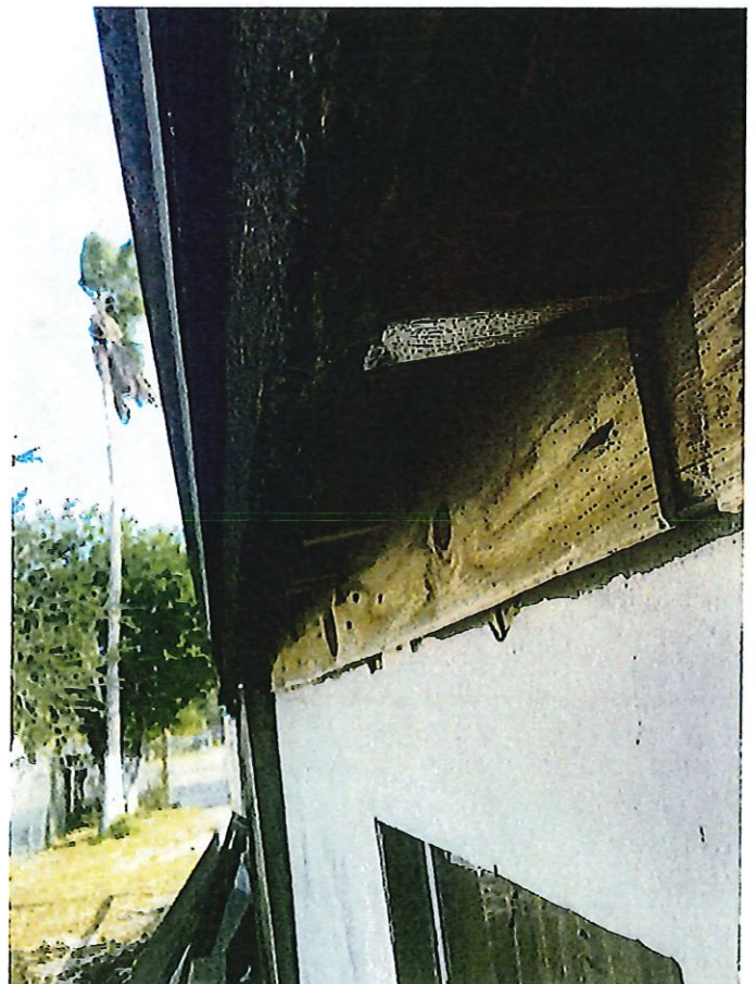
2x6 Rim board, Trim and Soffit severely damaged
