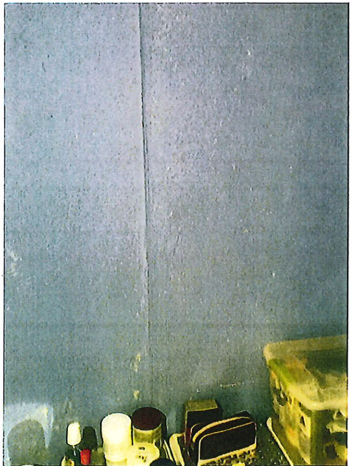
Crack in wall Second bedroom
