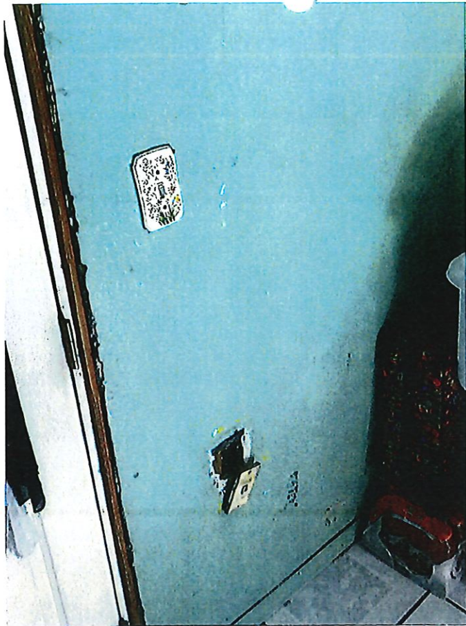
Sheet rock Damage
