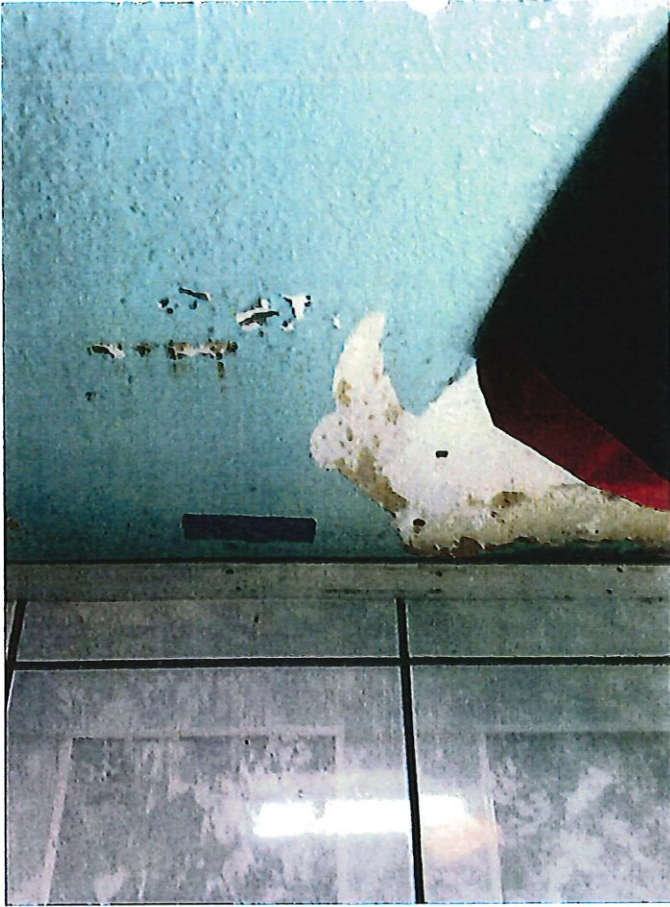
Master Bedroom water Damage from recent flooding
