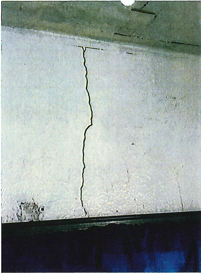
Crack above window in exterior CMU wall
