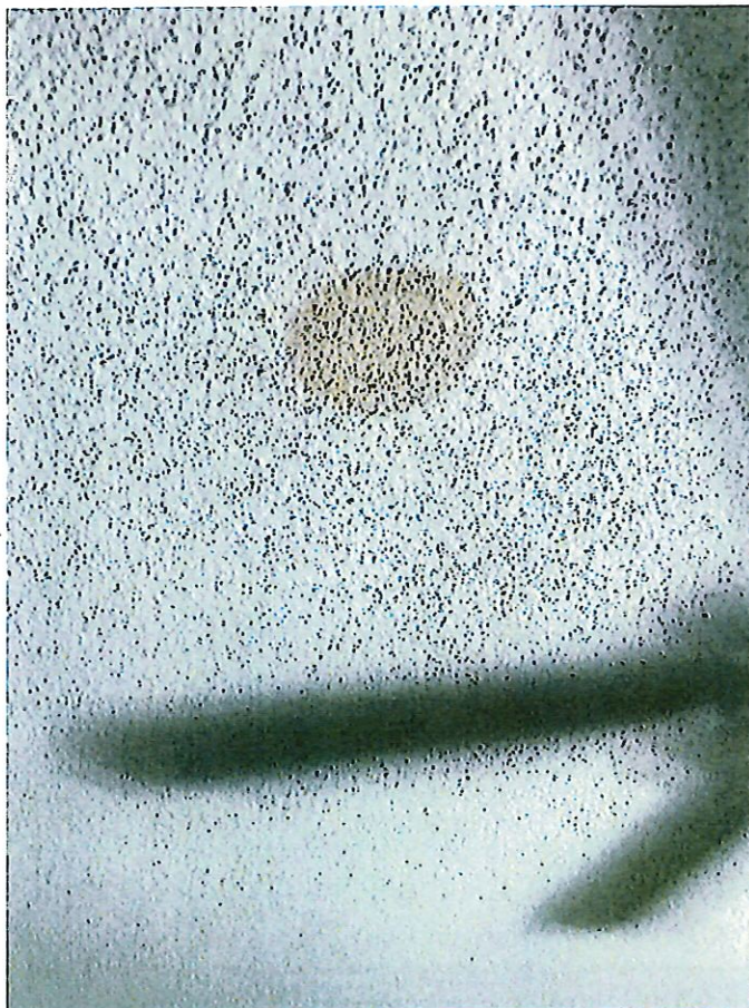
water staining on ceiling
