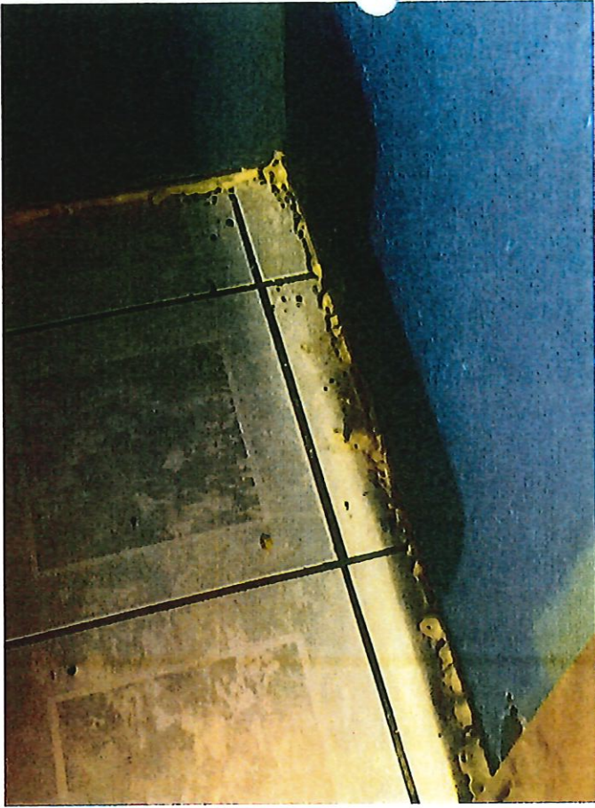
Separation of Floor and wall
