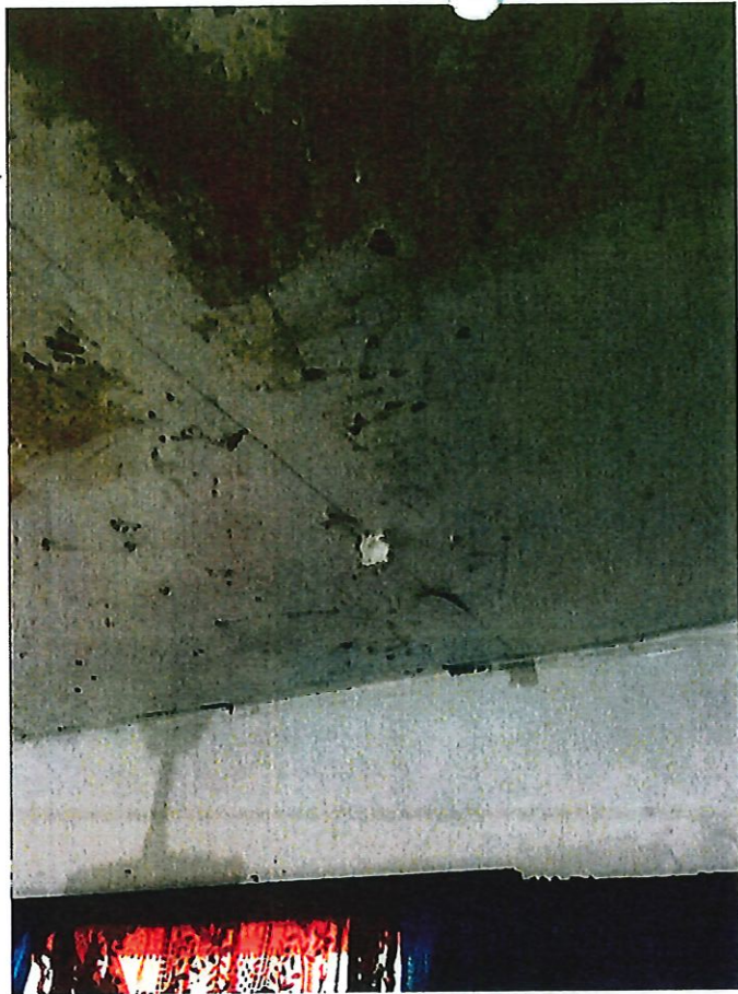
Water Damage to Ceiling in Living room
