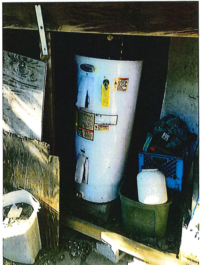
Water heater not protected from the elements
