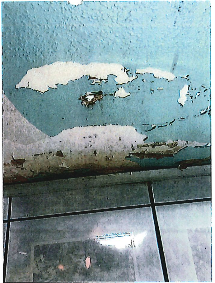
water Damage from recent flooding
