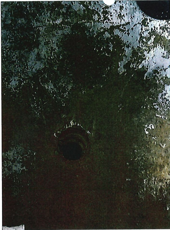
Shower Drain Does not work
