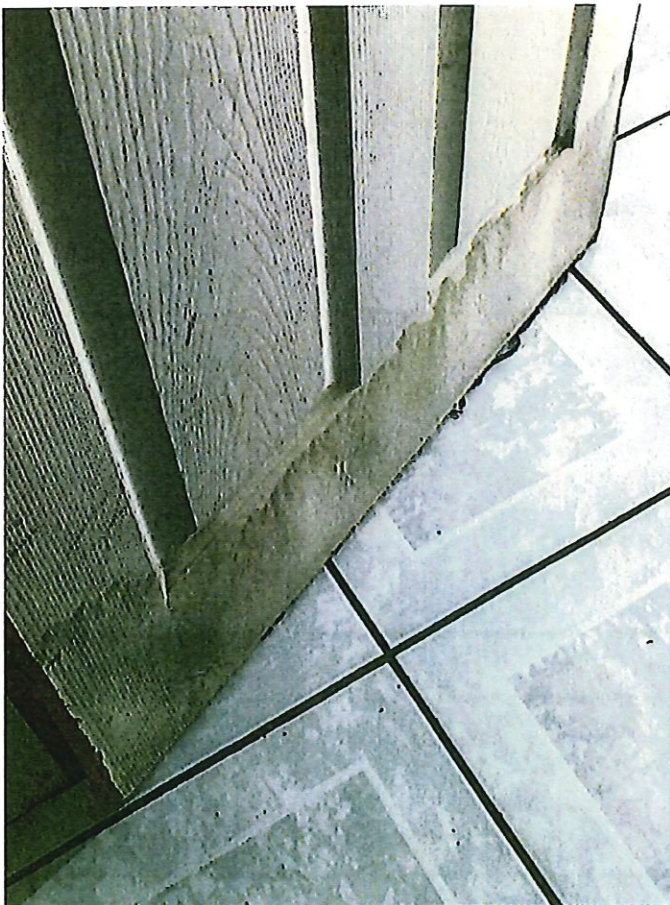
Water damage to door of Bedroom.
