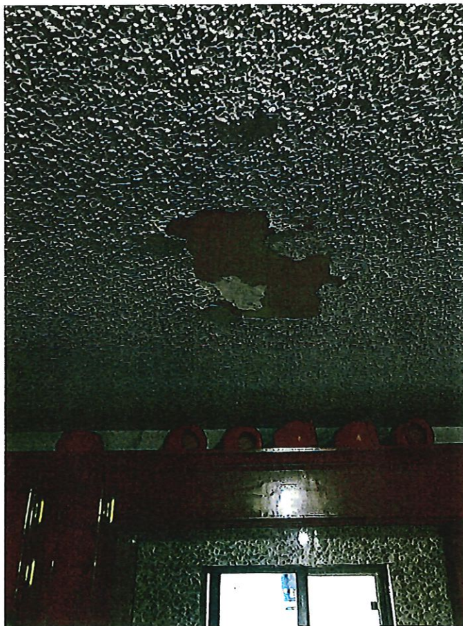
Texture peeling from ceiling
