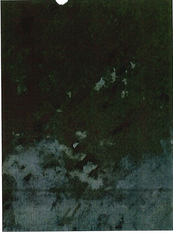
Water Damage close up
