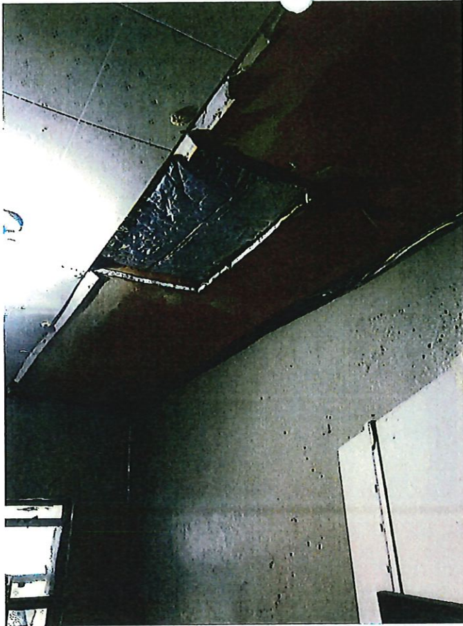
Water Damage in Restroom
