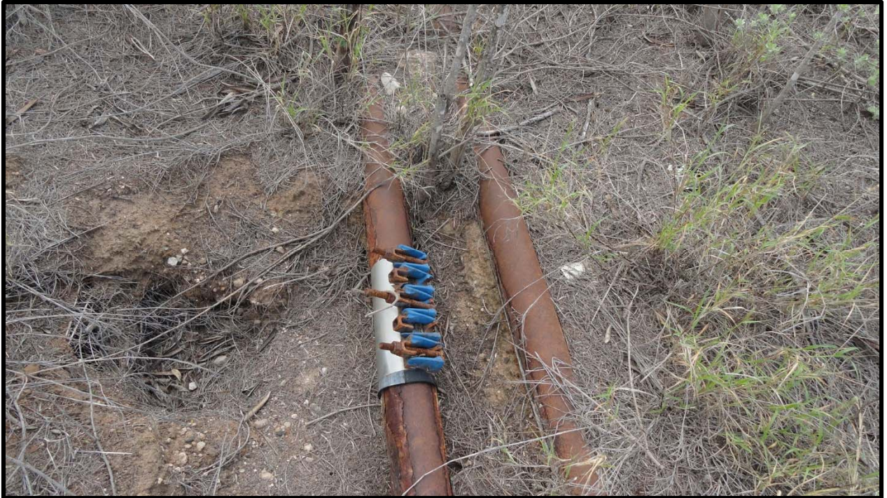
Out of use metal piping running from old stationary water pump, east to Iowa Road.
