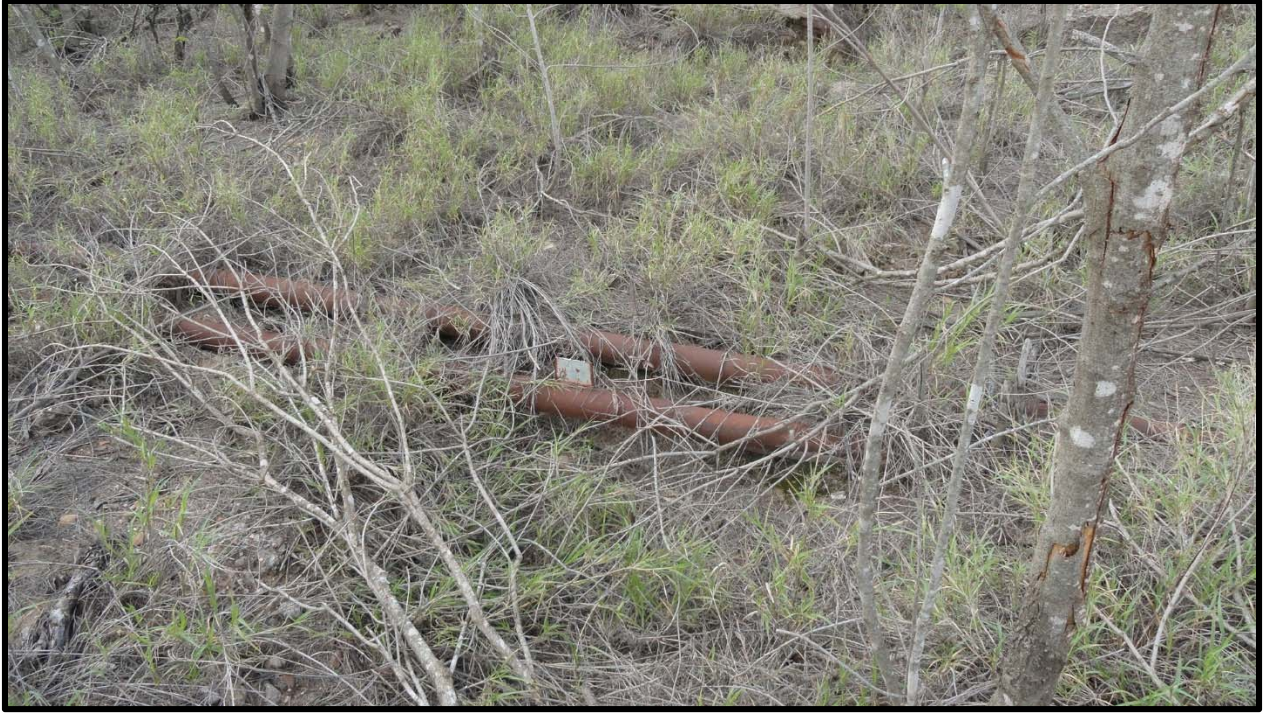
Out of use metal piping running from old stationary water pump, east to Iowa Road.
