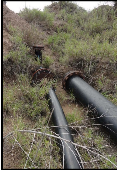
Water hose connection at Iowa Road.
