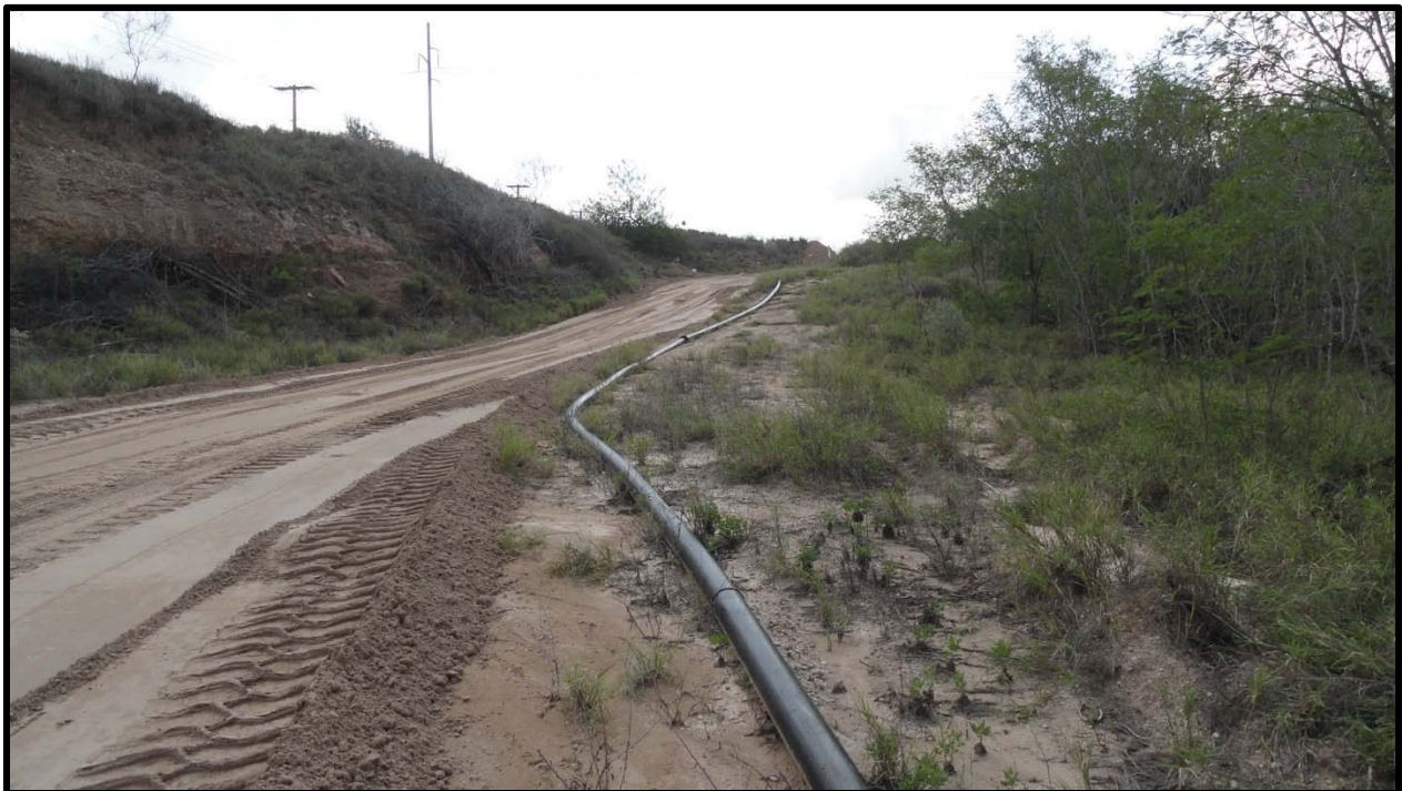
Plastic/rubber water hose along east access road to pump at Iowa Road.
