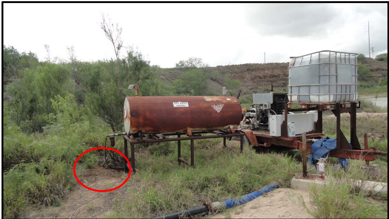
Diesel tank and mobile pump/generator at end of northeast access road.
