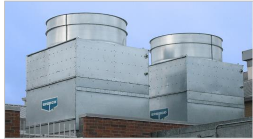
Equipment upgrades, like these new cooling towers, will result in lower energy consumption and lower O&M costs for the County.
