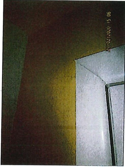
Cracks on walls
