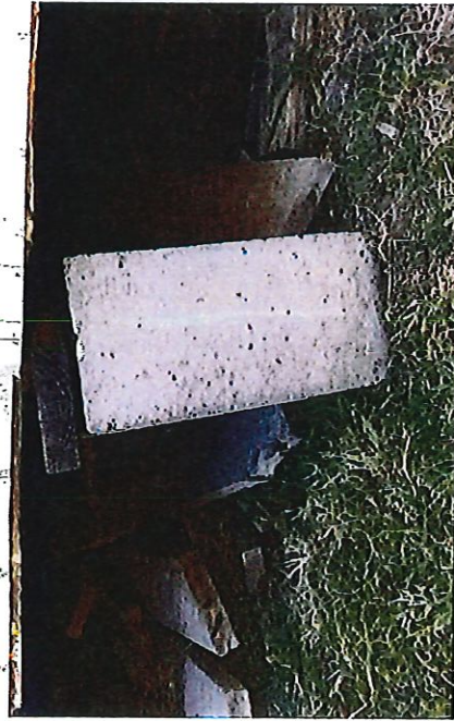
Pier and beams un even and leaning
