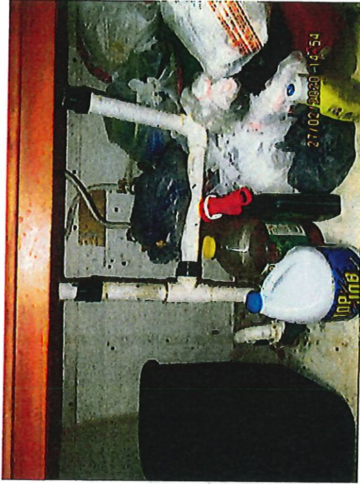
under sink inadequate plumbing joints
