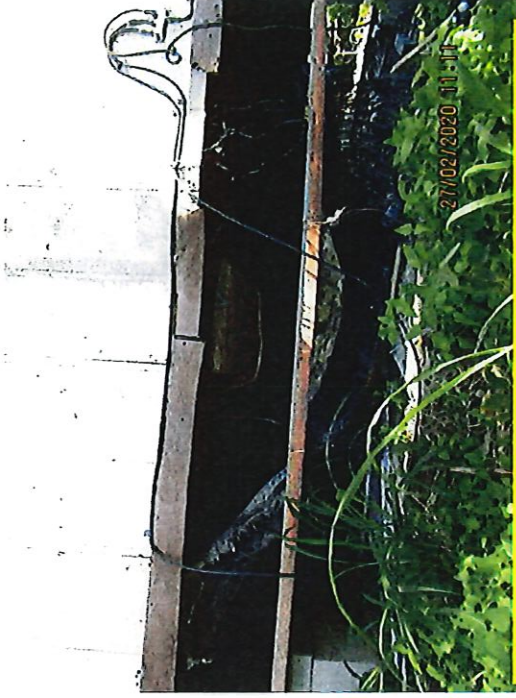
No Underpinning and floor insulation fallen to the ground
