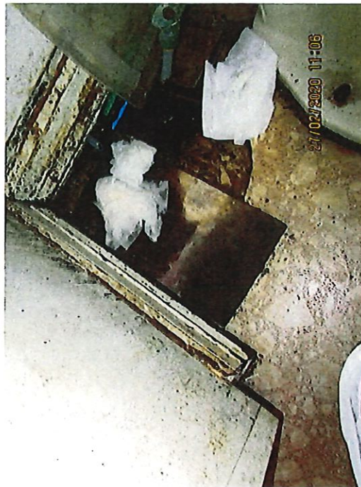
Mold and rot on base boards
